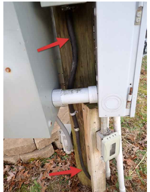
Circuit wiring not protected in conduit.
