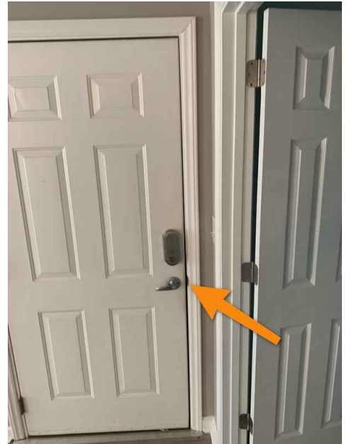
Passage lock does not latch at front entry door.
