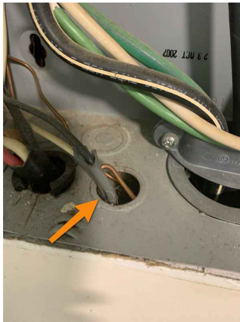
Laundry sub panel box.
