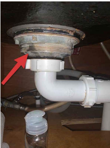
Left sink drain leaking under kitchen sink.
