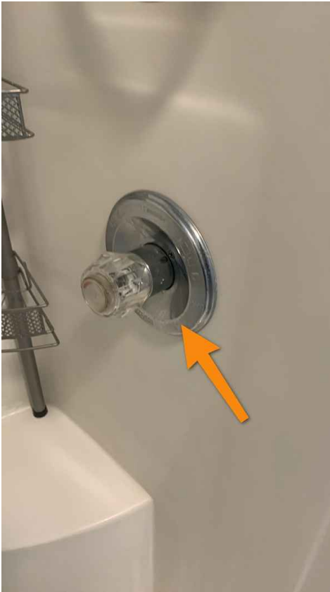
Shower faucet loose.
