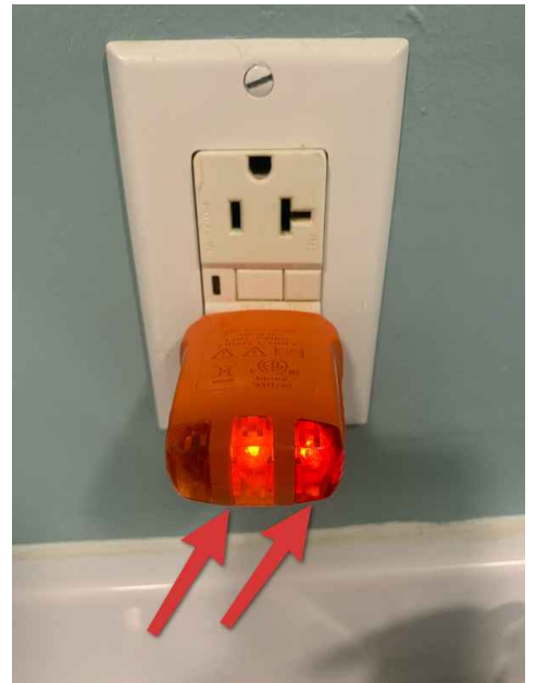
Light pattern indicates hot and neutral reversed at bathroom GFCI receptacle.
