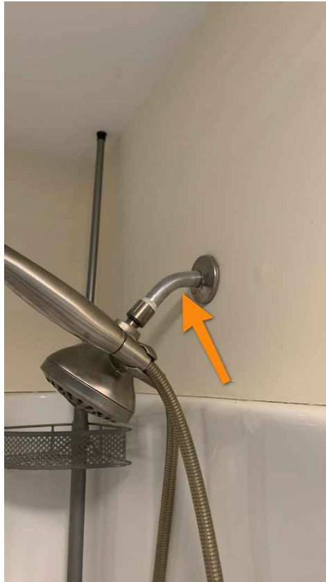
Shower arm post loose.
