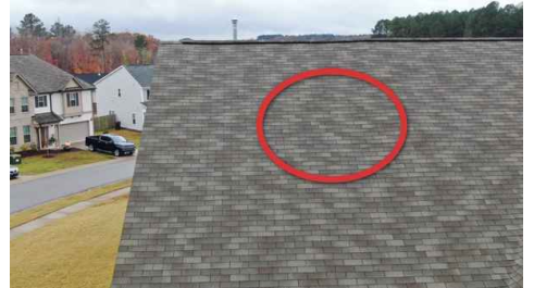
Front side of roof, some tabs with minor lifting
