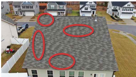
Rear side of the house Various Areas, minor lifting
