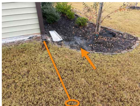
Front Left Exterior, arrow showing washout
