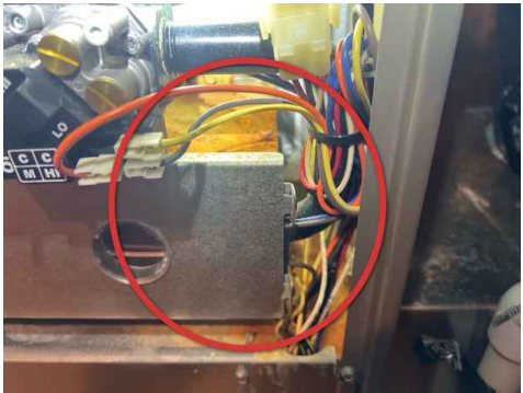
Furnace on heat exchanger box
