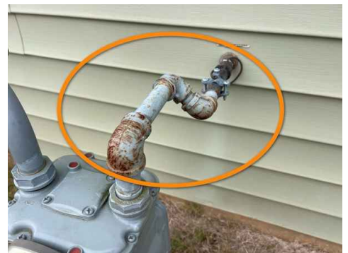
Gas supply, outlet side of meter
