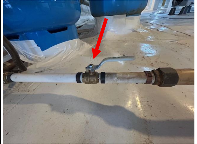
Pressure storage tank shut off vavle shown
