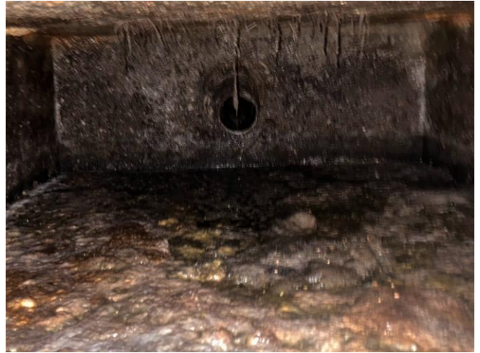
Inlet side shown from the outlet inspection port - root intrusion shown around the inlet inspection port.
