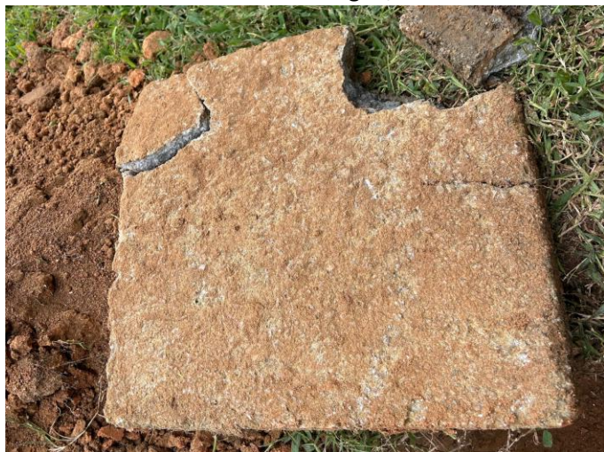
Distribution box lid shown damaged/deteriorated.
