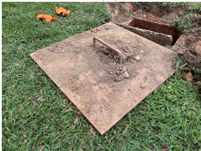
Outlet riser fitted with an improper lid.
