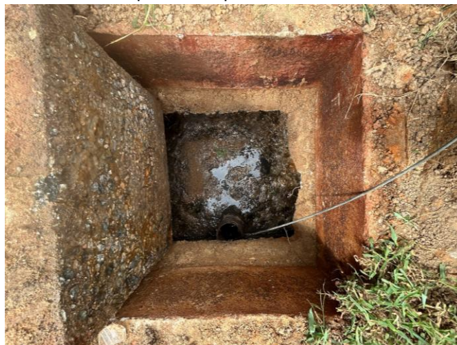
Outlet shown open for inspection.
