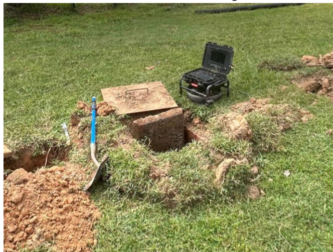
Outlet riser shown less than 3" above grade.
