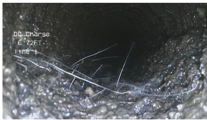
Drain line 1 shown scoped with accumulated solids and root intrusion.
