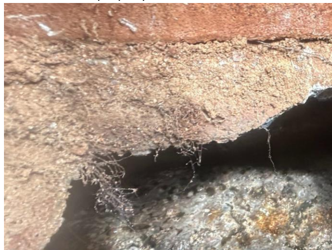
Root intrusion shown around outlet inspection port - outlet riser not properly sealed to tank.
