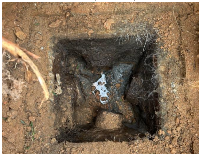
Distribution box shown open for inspection.
