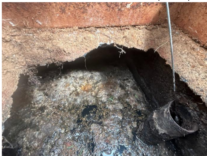
Deterioration shown around the outlet inspection port.
