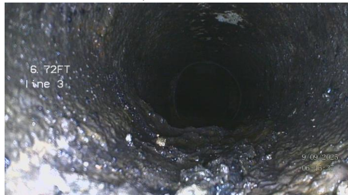
Drain line 3 shown scoped with accumulated solids.
