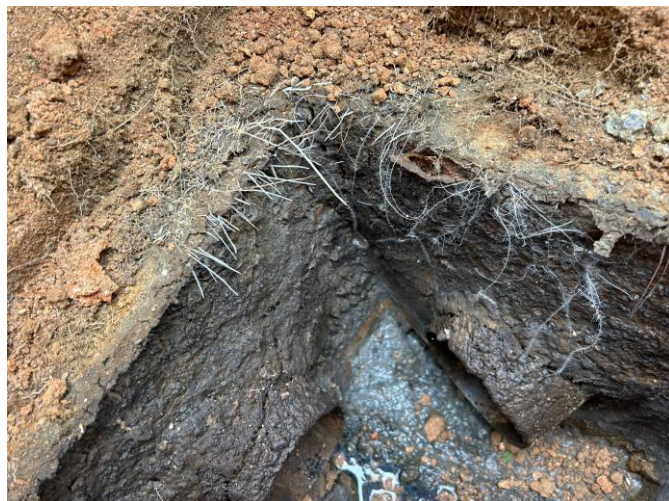
Root intrusion shown in the distribution box.
