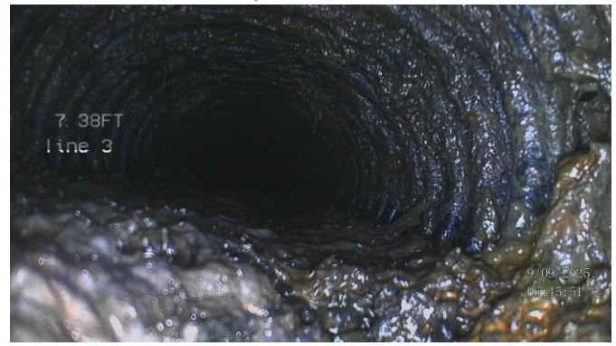
Drain line 3 shown scoped with accumulated solids.
