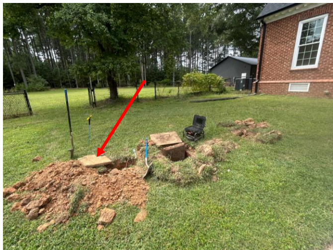
Distribution box location shown.
