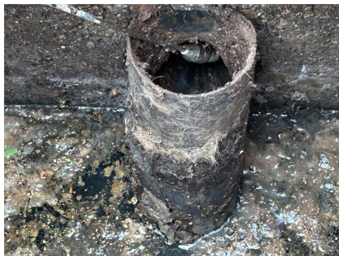
Effluent level shown at least 5" below a normal effluent level.
