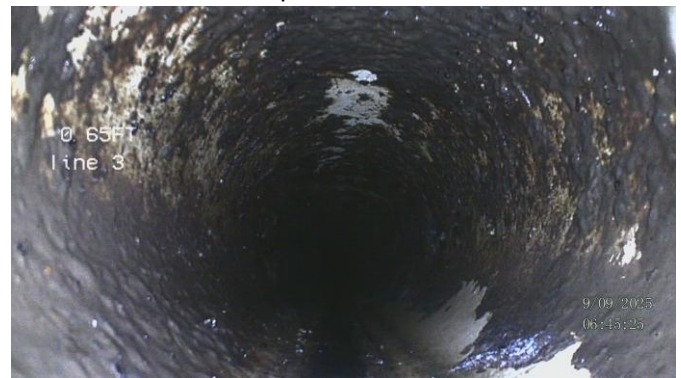
Drain line 3 shown scoped with accumulated solids.
