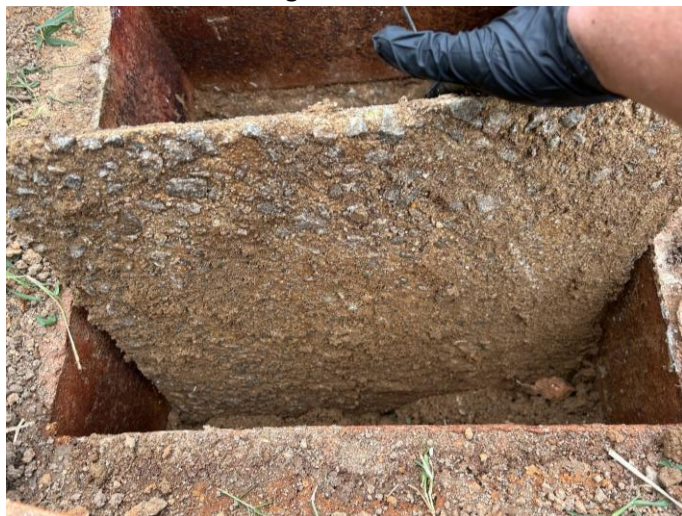
Outlet lid shown missing a handle
