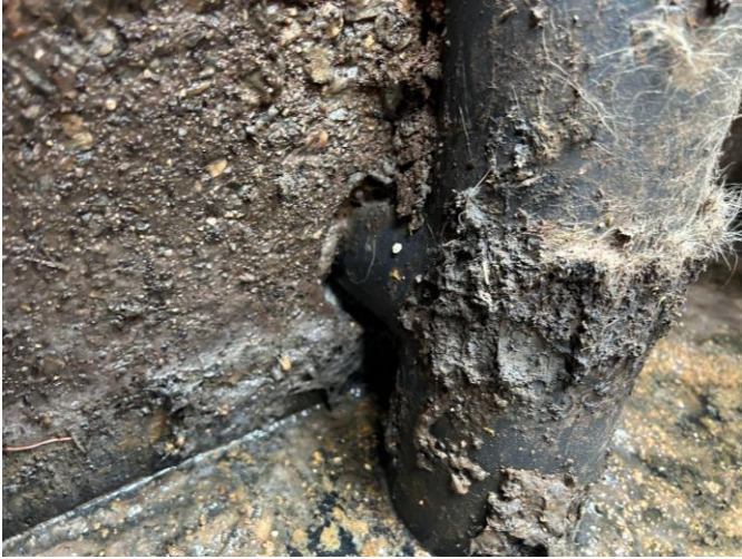
Outlet pipe penetration shown not properly sealed.
