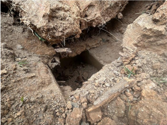
Inlet riser shown damaged.
