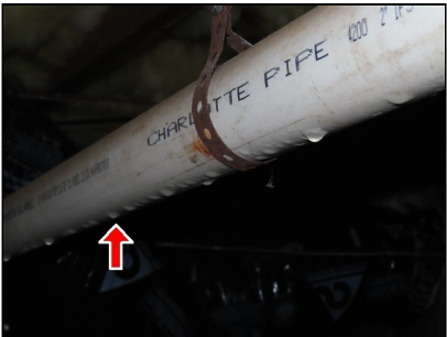
condensation on plumbing pipes
