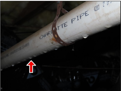
condensation on plumbing pipes
