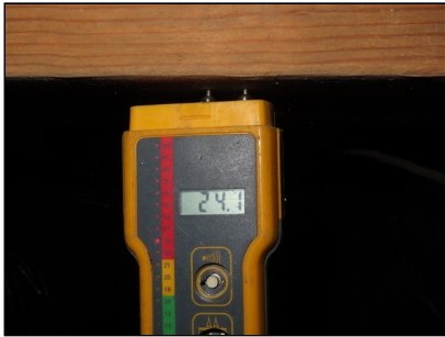
framing moisture over 24%
