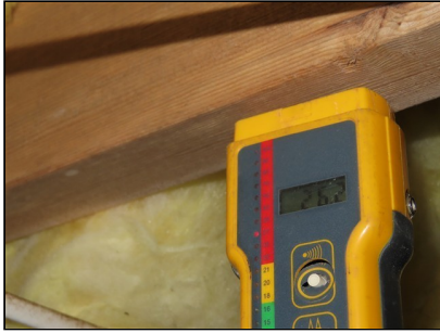
framing moisture over 26%
