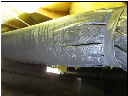
condensation on ductwork
