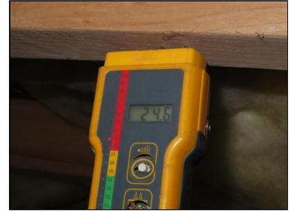
framing moisture over 24%
