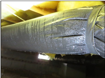
condensation on ductwork
