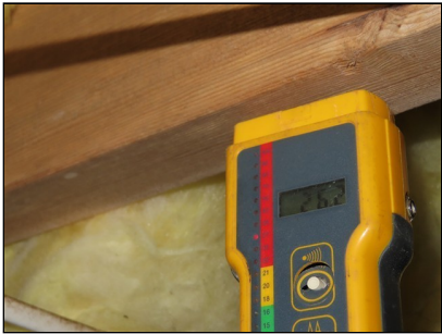
framing moisture over 26%
