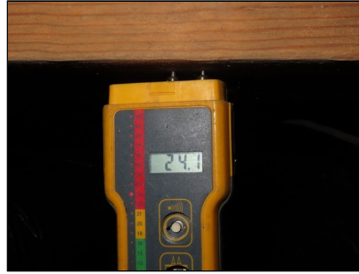
framing moisture over 24%
