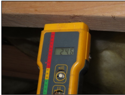
framing moisture over 24%
