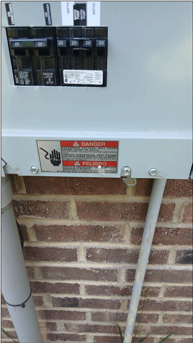
7.0 DISTRIBUTION PANEL (Picture 2)
