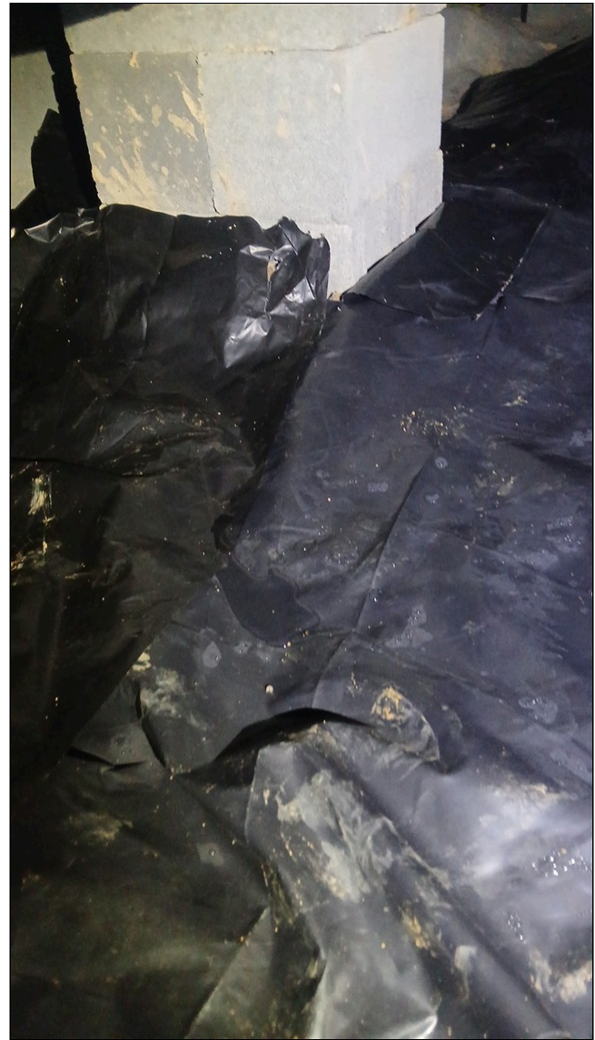
12.1 INTERIOR CONDITIONS / SIGNN OF WATER INTRUSION (Picture 2)
