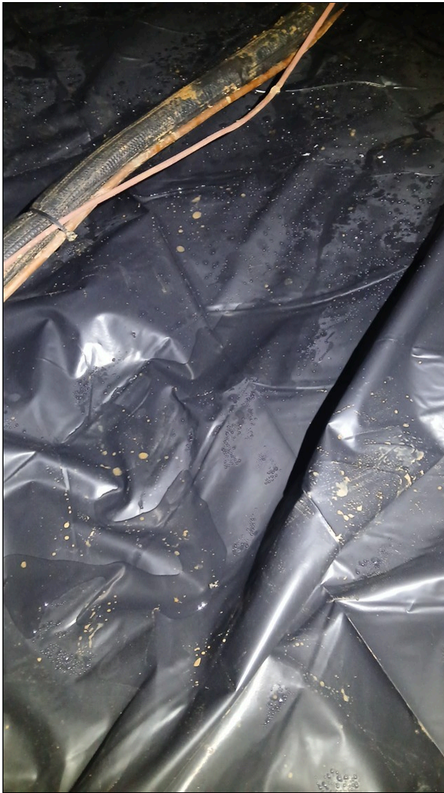
12.1 INTERIOR CONDITIONS / SIGNN OF WATER INTRUSION (Picture 1)
