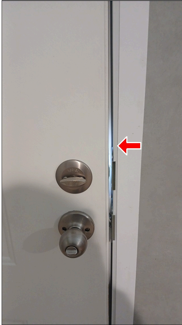
2.2 (2) Rear exterior door knob is loose. Due to security concerns recommend to secure.
