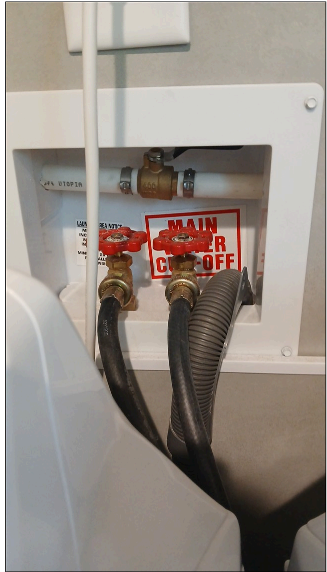
9.0 MAIN WATER CUTOFF (Picture 2)
