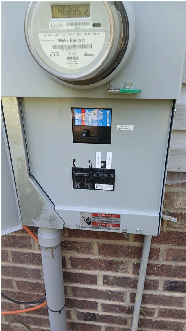
7.0 DISTRIBUTION PANEL (Picture 1)
