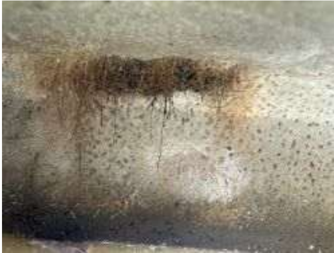
Baffle wall with root intrusion.
