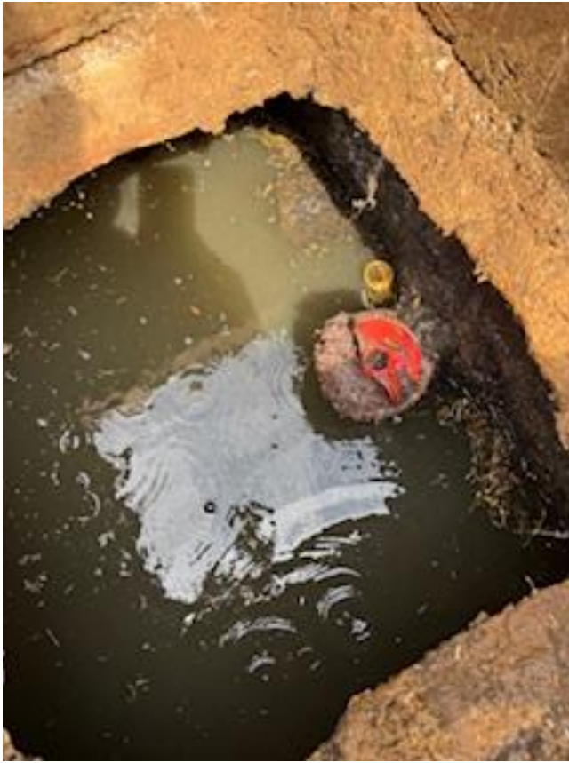
TANK OUTLET TEE AND FILTER
