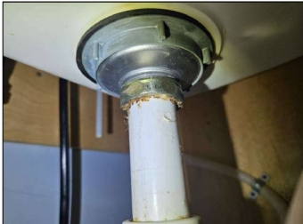
There is a leak in the drain plumbing at the kitchen sink.
