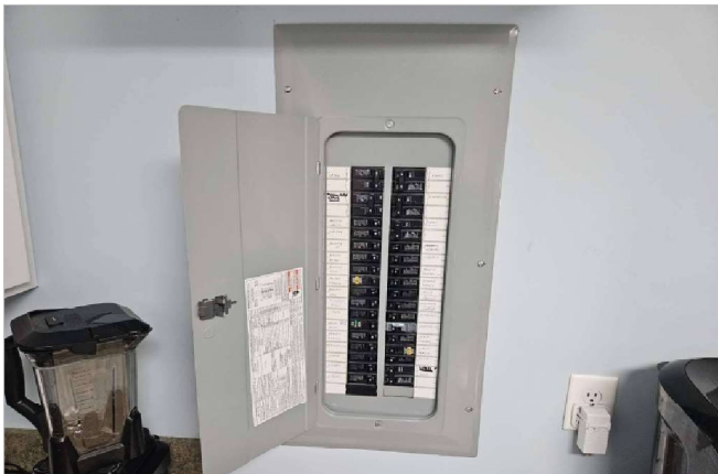
The home sub-electrical panel is located in the laundry area.
