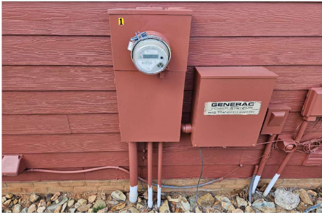
The electrical service entrance and main electrical panel are located at the right elevation.
