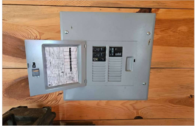
The small outbuilding electrical panel is located inside the building.
