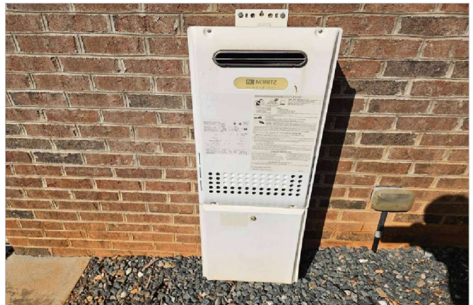
The water heater is located at the rear elevation of the home.
