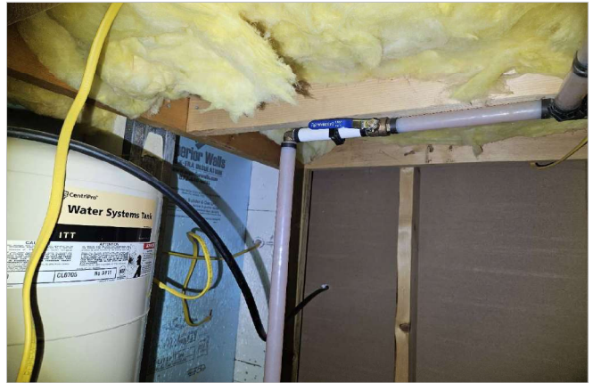
The main water shutoff is located in the garage near the pressure tank.
