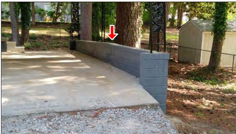
1.0 Item 10(Picture) Heaving foundation wall
