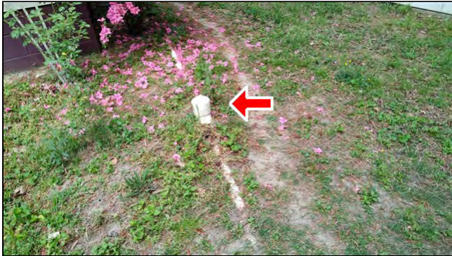
5.6 Item 1(Picture) Plumbing cleanout not trimmed
