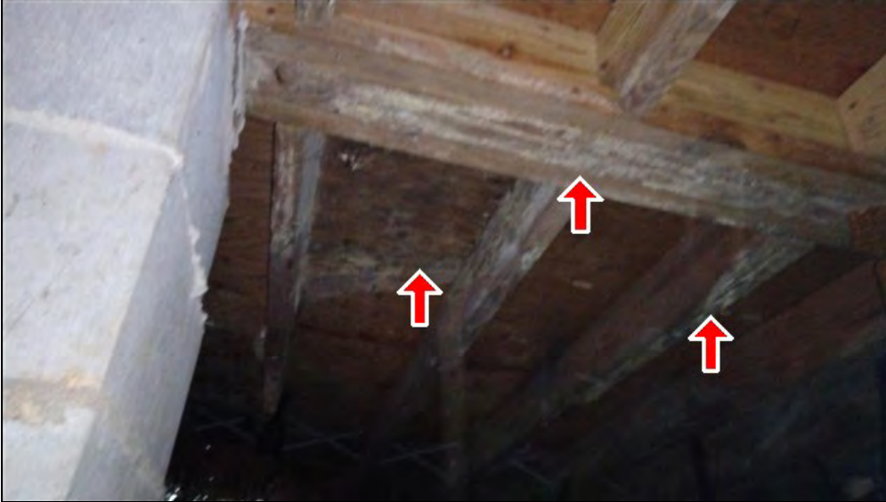
1.2 Item 1(Picture) The floor framing has fungal growth with some deterioration noted
