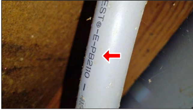
5.1 Item 1(Picture) Polybutylene Piping noted in the home
