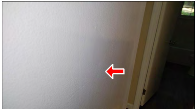
4.4 Item 2(Picture) Holes with improper repairs noted
