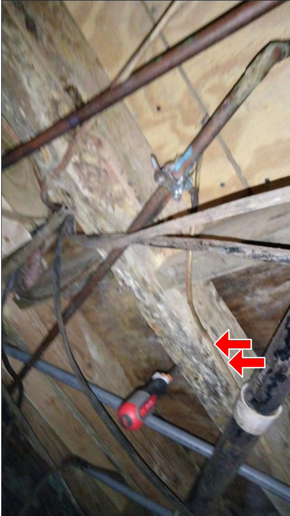
1.2 Item 5(Picture) Deteriorated floor joist noted
