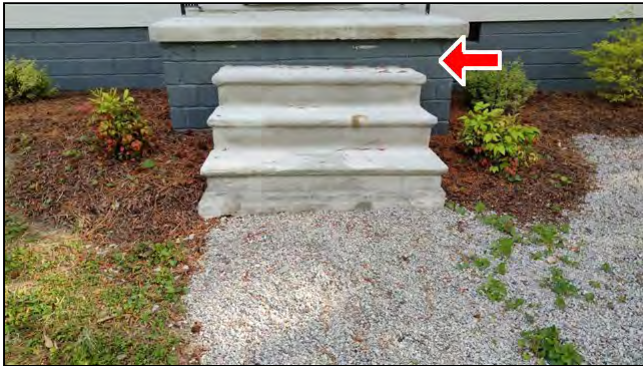
2.6 Item 1(Picture) The front steps have settled
