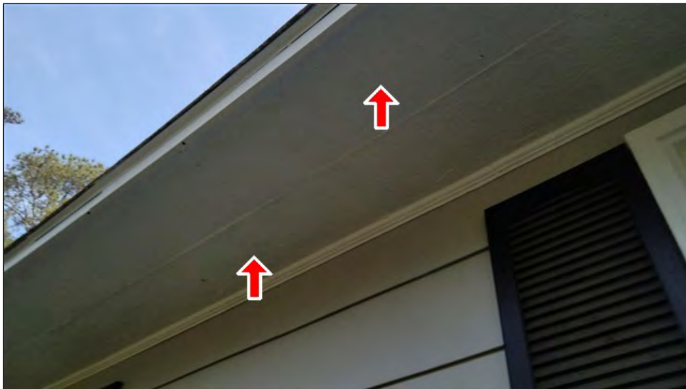
2.1 Item 1(Picture) Soffits are not a exterior grade material
