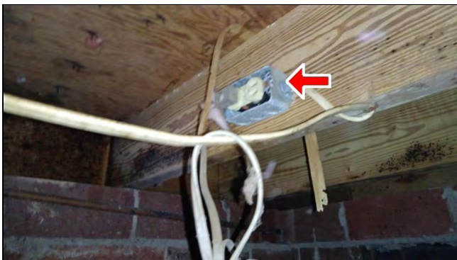
5.7 Item 1(Picture) Sump pump is not powered by a GFCI for protection
