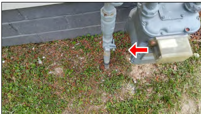
10.3 Item 2(Picture) The gas is off to the home
