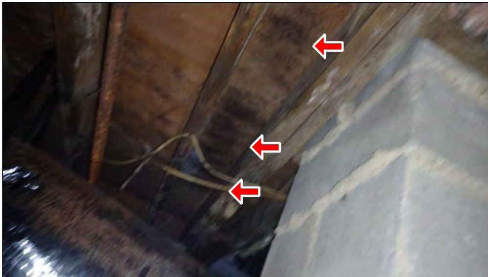
1.2 Item 9(Picture) Fungal growth with deterioration noted
