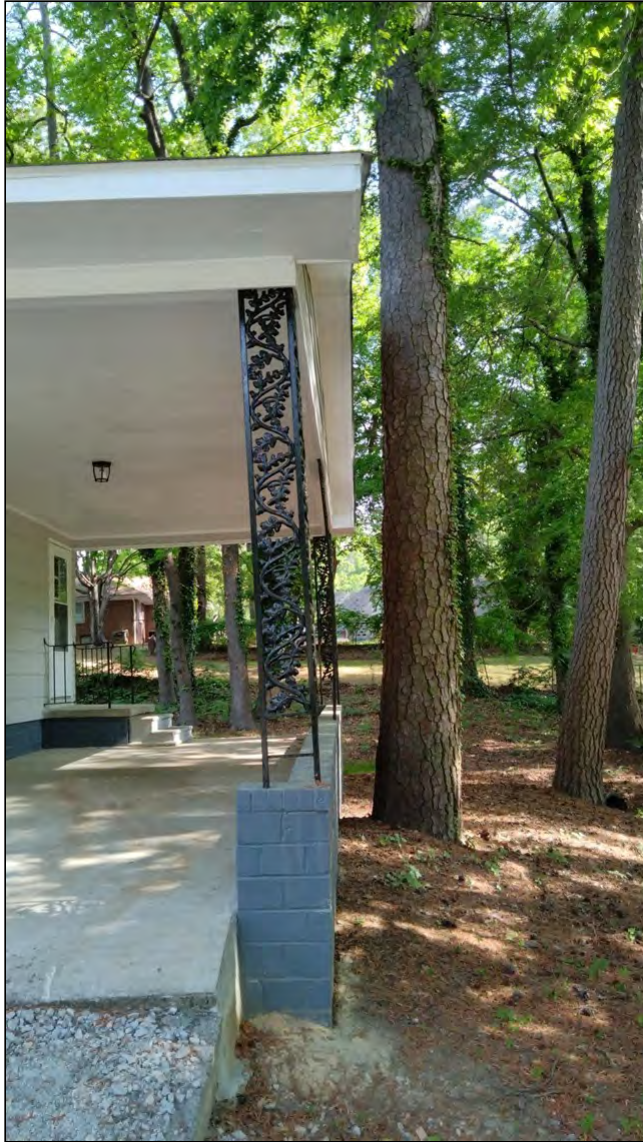
1.0 Item 12(Picture) Leaning foundation wall
