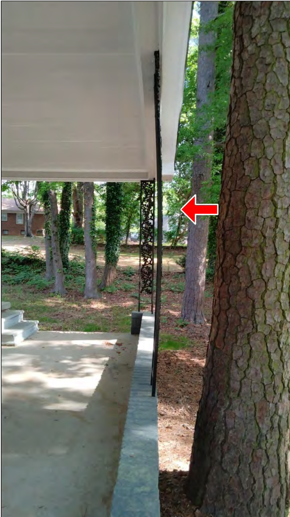
1.0 Item 11(Picture) Leaning and heaving carport foundation wall
