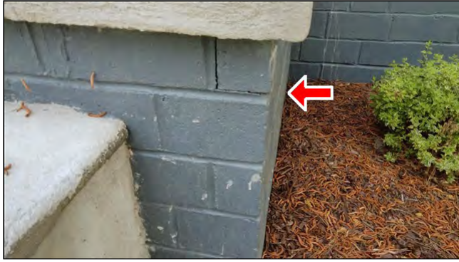
1.0 Item 1(Picture) Common cracks in the mortar joints
