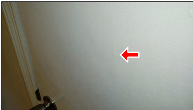
4.4 Item 1(Picture) Holes with improper repairs noted
