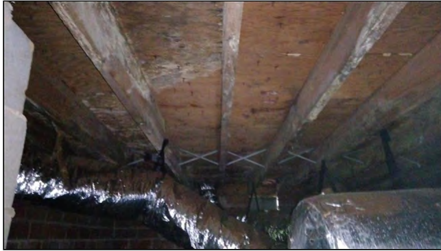
11.1 Item 1(Picture) Missing flooring insulation
