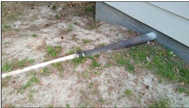
5.6 Item 2(Picture) Plumbing waste line is exposed in the yard
