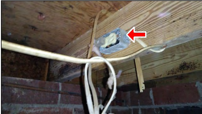
8.5 Item 1(Picture) Receptacle cover missing
