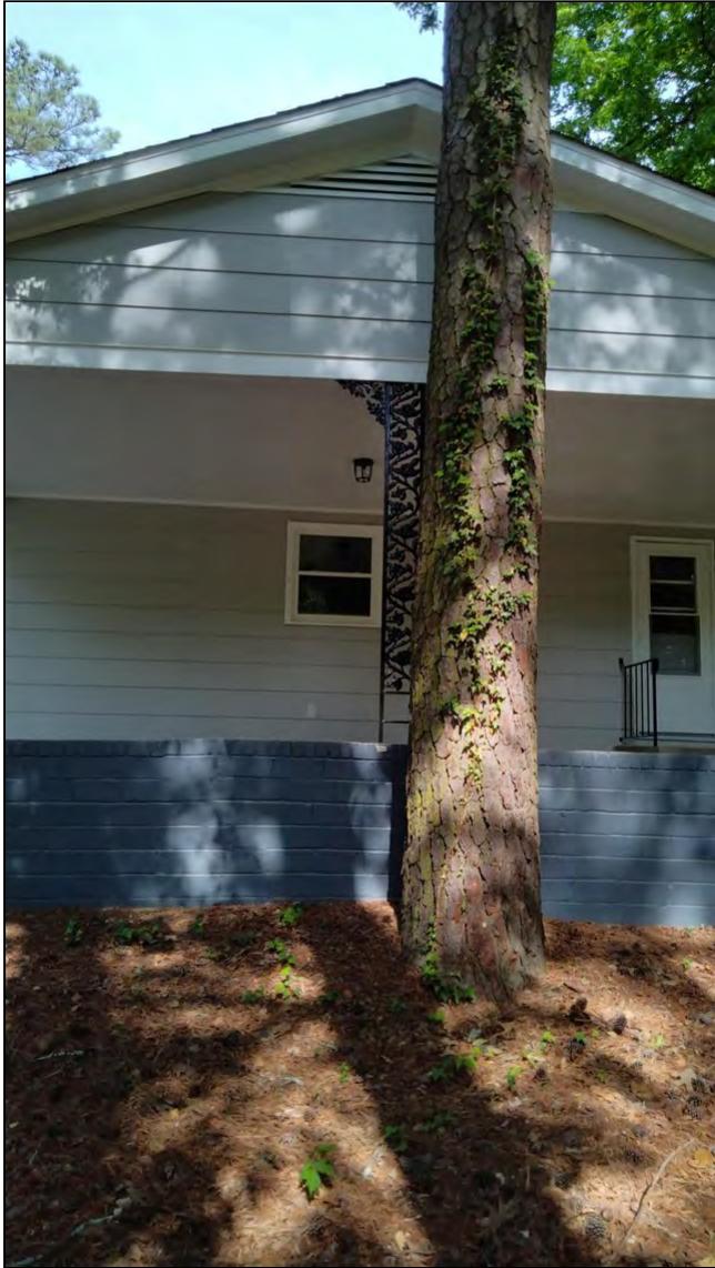
1.0 Item 6(Picture) A very large pine tree is growing against the foundation and the tree roots are causing damaged to the foundation
