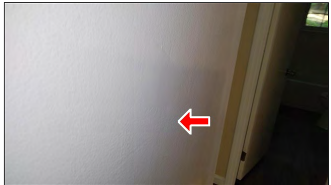
4.4 Item 2(Picture) Holes with improper repairs noted
