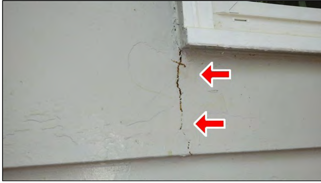
2.0 Item 3(Picture) Damaged siding noted
