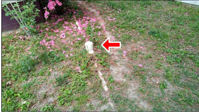
5.6 Item 1(Picture) Plumbing cleanout not trimmed
