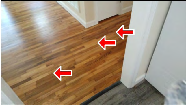
4.2 Item 1(Picture) Raised area in the flooring
