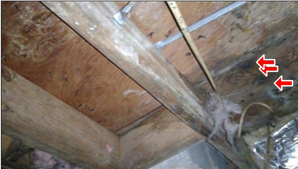
1.2 Item 8(Picture) Deteriorated sheathing noted
