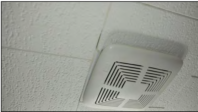
4.0 Item 1(Picture) Damaged ceiling tile
