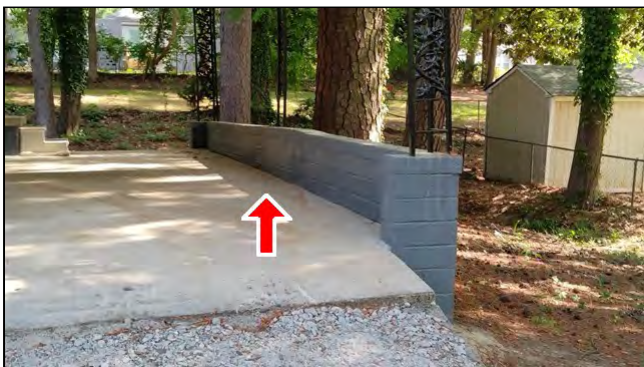
1.0 Item 4(Picture) Up heaving in the carport foundation wall
