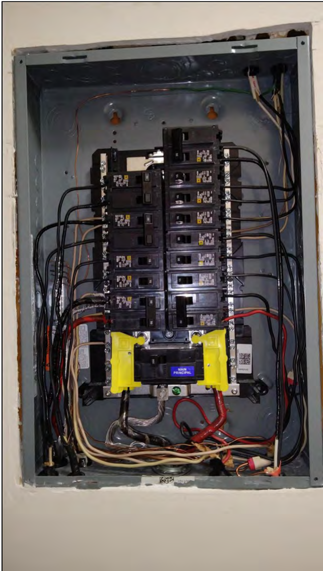
8.2 Item 1(Picture) The main electrical panel
