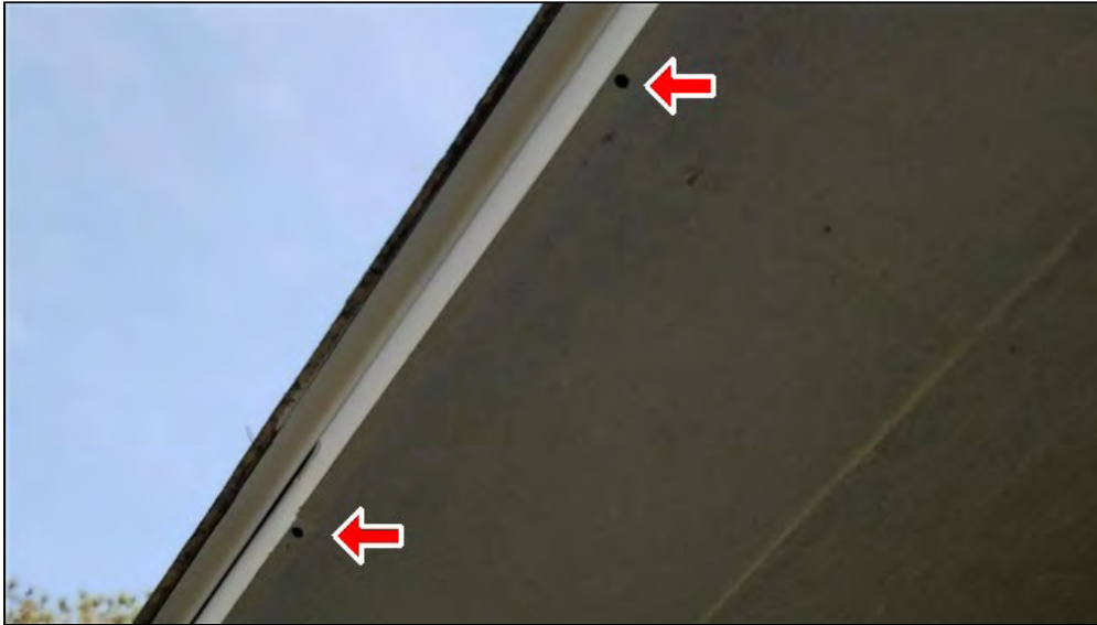
2.1 Item 2(Picture) Insect damage noted to the fascia boards
