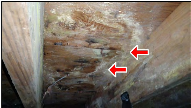
1.2 Item 2(Picture) Fungal growth noted
