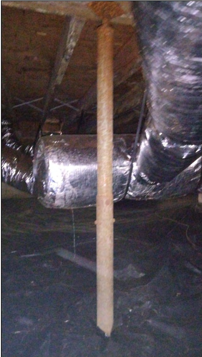
1.1 Item 1(Picture) Metal stand pier with no or improper footers
