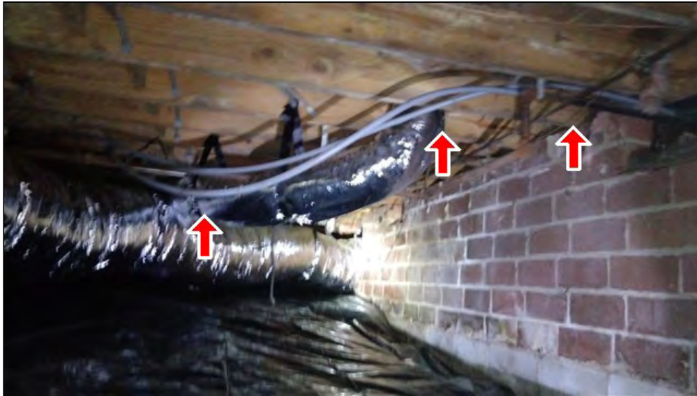
5.1 Item 2(Picture) Polybutylene piping noted
