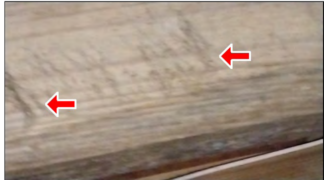
1.2 Item 3(Picture) Fungus growth on the floor joists
