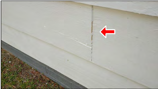
2.0 Item 4(Picture) Loose siding. Moves to the touch
