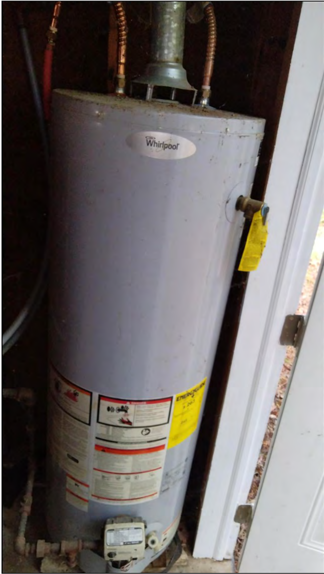
6.0 Item 1(Picture) The water heater
