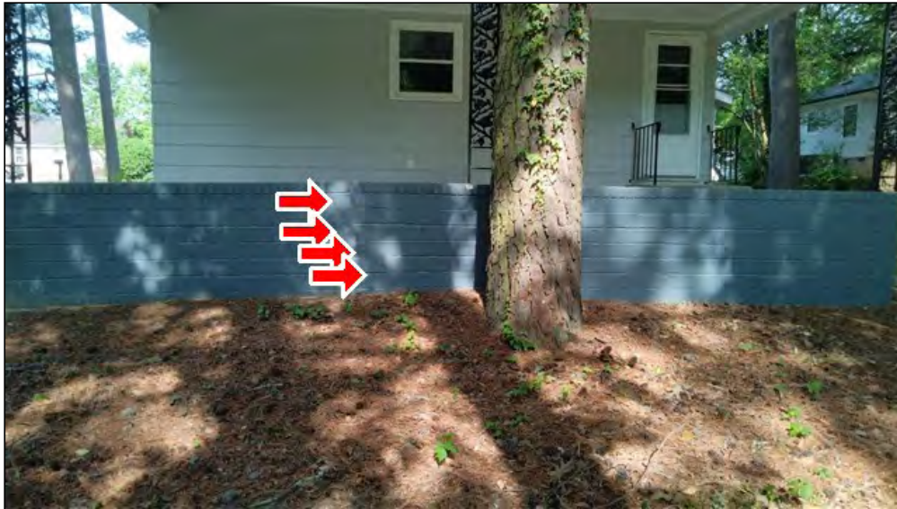
1.0 Item 7(Picture) Structural cracks in the carport foundation wall next to the large tree
