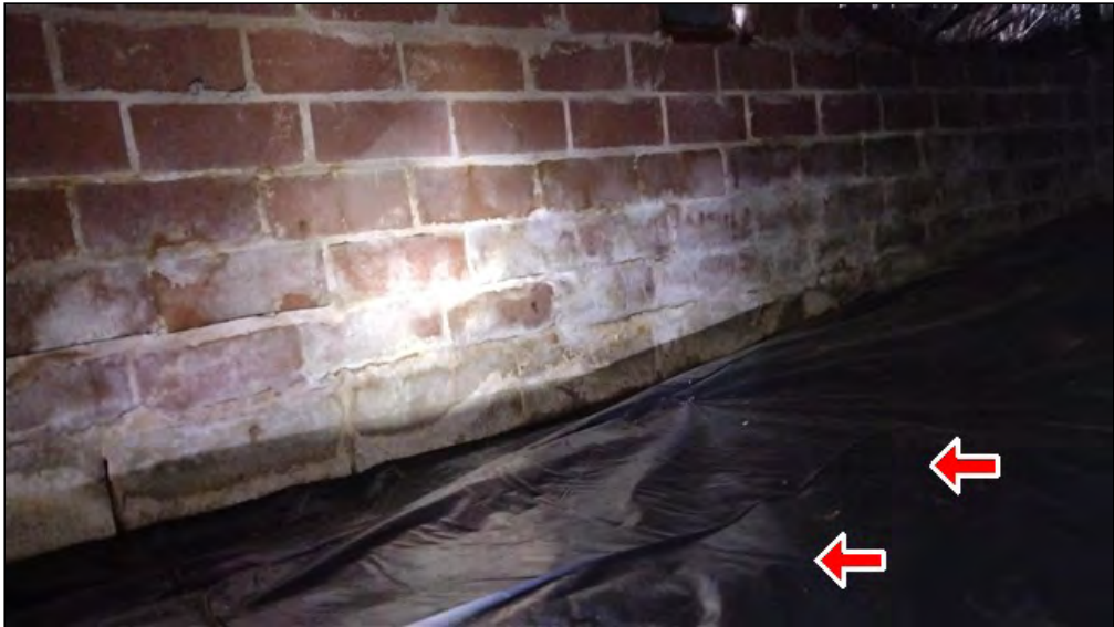
11.2 Item 1(Picture) Plastic vapor barrier
