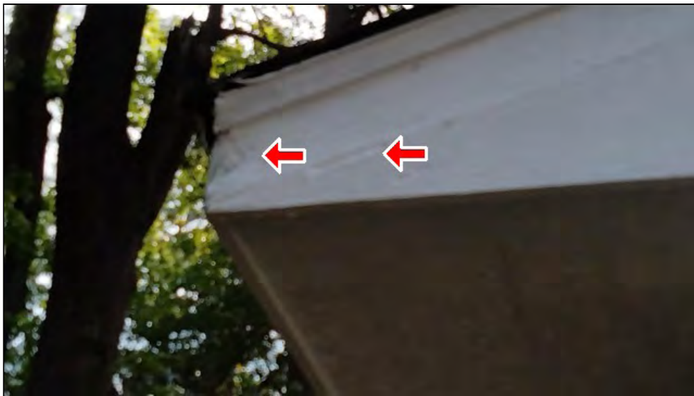
2.1 Item 3(Picture) Deterioration / damage noted
