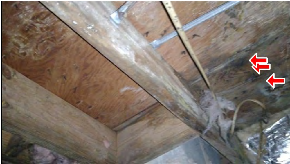
1.2 Item 8(Picture) Deteriorated sheathing noted
