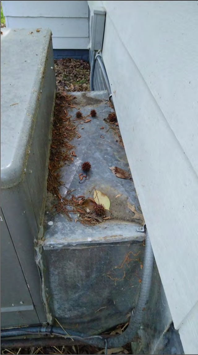
10.3 Item 1(Picture) Metal holding water and rusting
