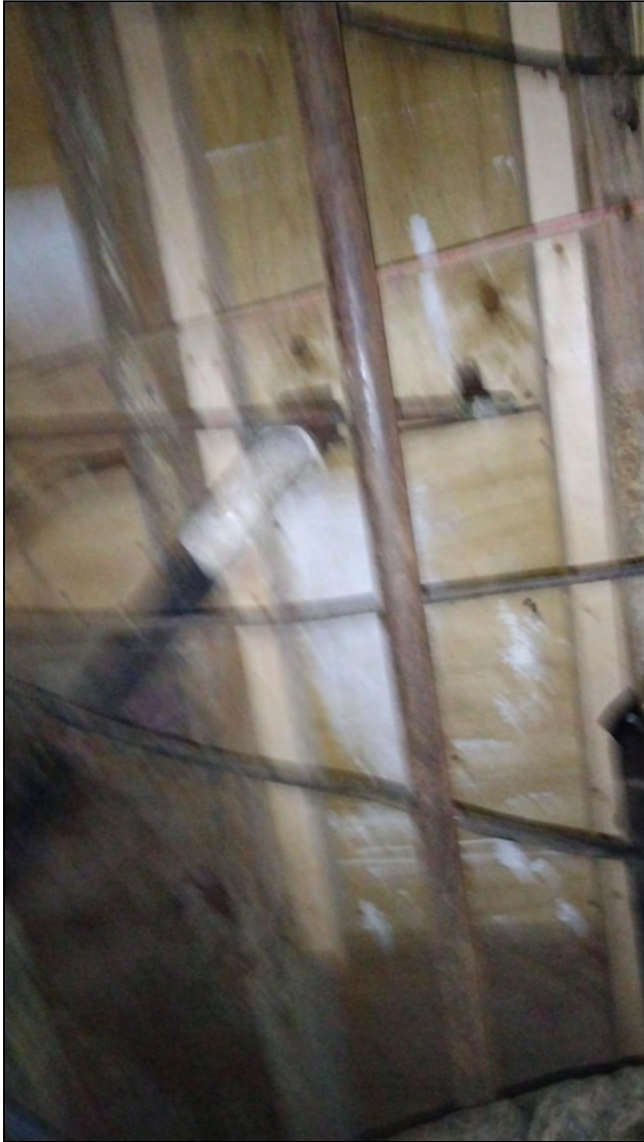
1.2 Item 6(Picture) Areas under the bathroom has been replaced in the past
