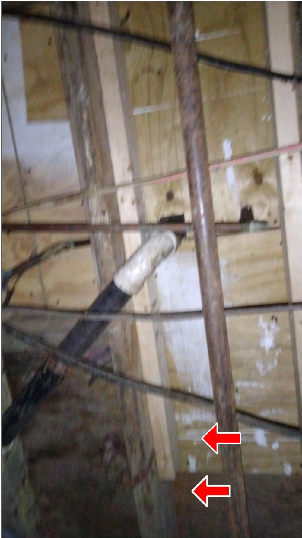
1.2 Item 10(Picture) The new floor joist is nailed to the deteriorated joist and is not supported to the ends
