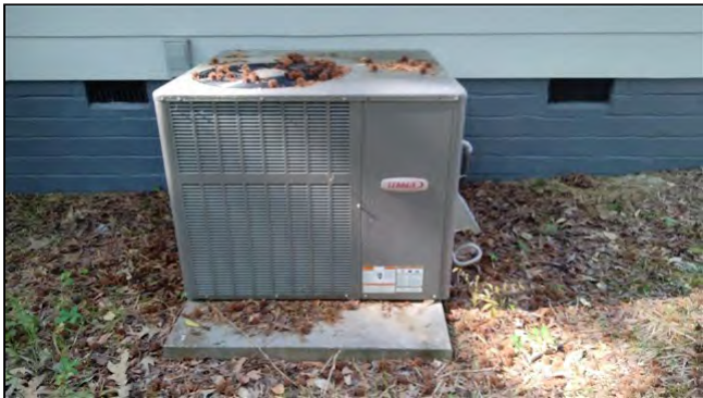
9.0 Item 1(Picture) The gas package unit
