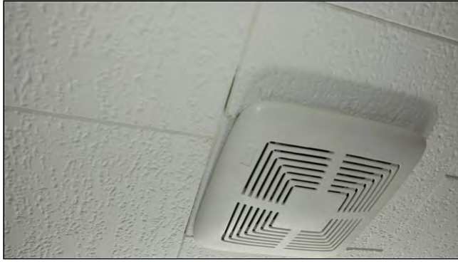
4.0 Item 1(Picture) Damaged ceiling tile
