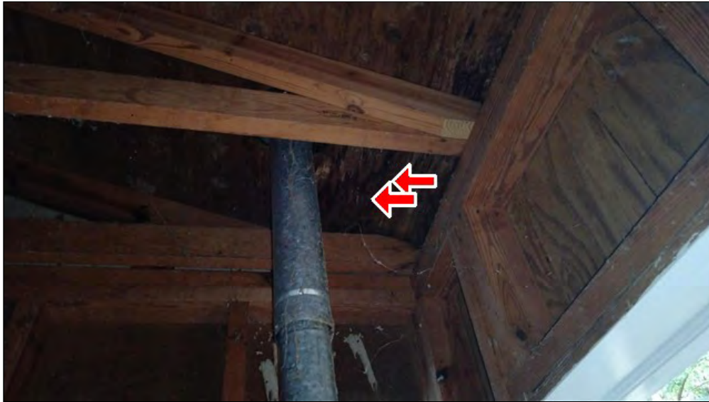
1.8 Item 1(Picture) Deteriorated sheathing noted in the storage room
