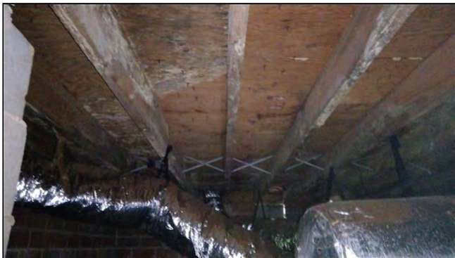
11.1 Item 1(Picture) Missing flooring insulation
