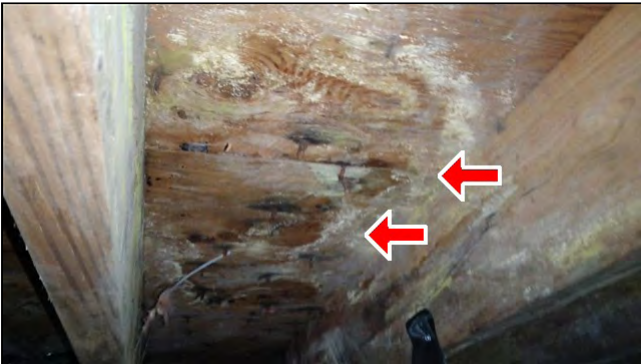
1.2 Item 2(Picture) Fungal growth noted
