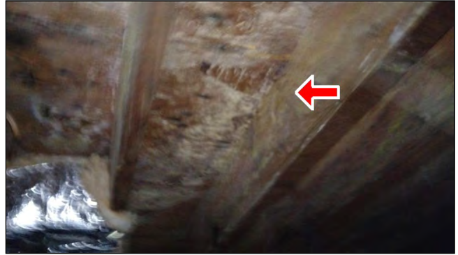
1.2 Item 7(Picture) Fungal growth on the floor sheathing
