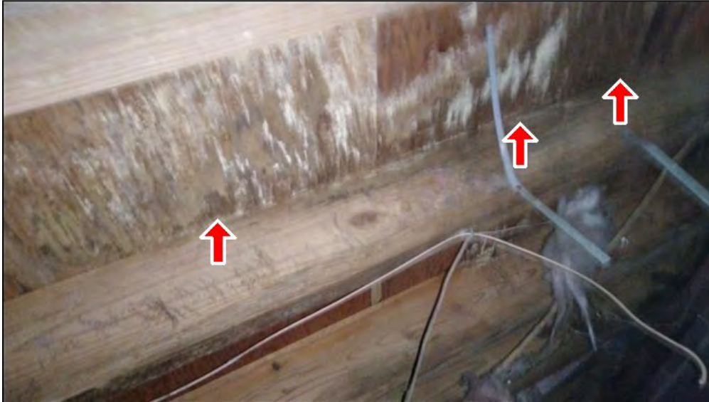
1.2 Item 4(Picture) Deteriorated floor sheathing and fungal growth
