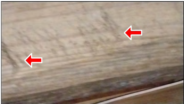
1.2 Item 3(Picture) Fungus growth on the floor joists
