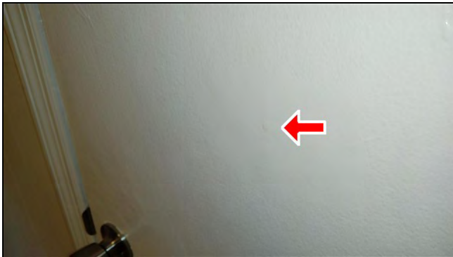
4.4 Item 1(Picture) Holes with improper repairs noted
