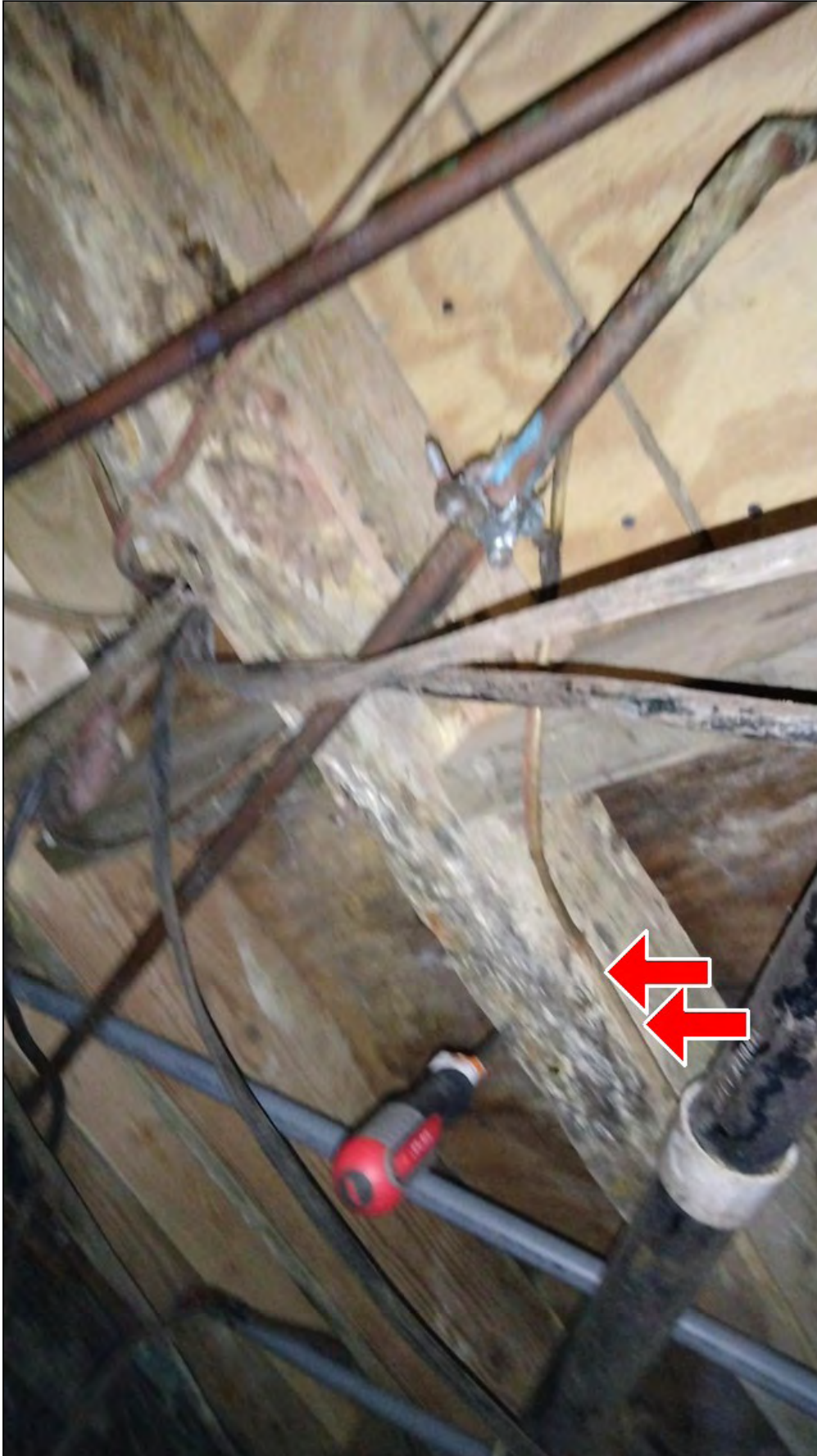
1.2 Item 5(Picture) Deteriorated floor joist noted
