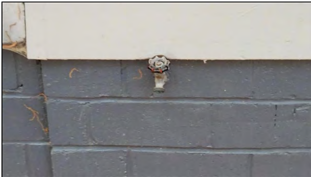
5.2 Item 1(Picture) Loose hose bib noted
