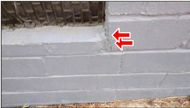
1.0 Item 3(Picture) Common cracks noted in the foundation at the foundation vents
