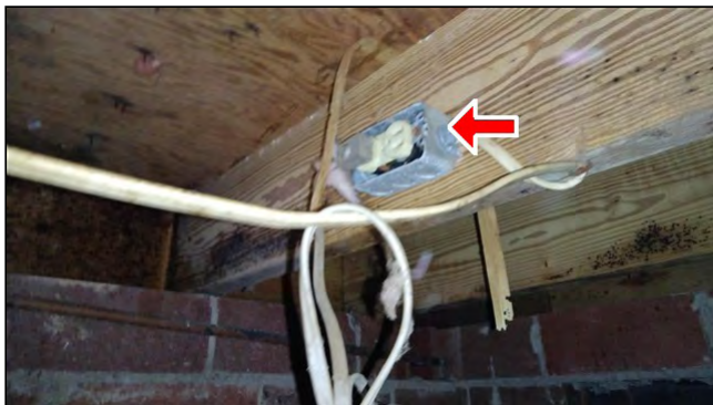
8.5 Item 1(Picture) Receptacle cover missing
