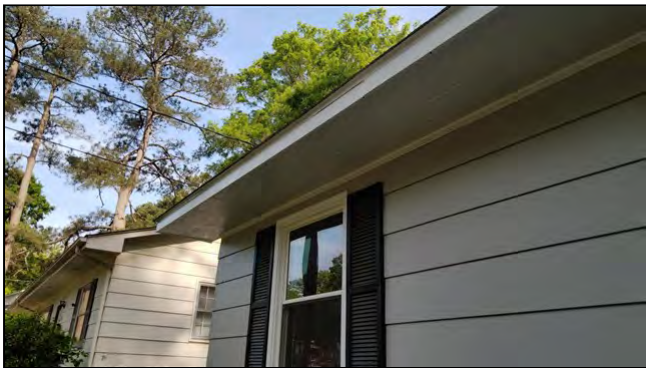
3.1 Item 1(Picture) No gutters are on the home
