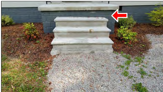
2.6 Item 1(Picture) The front steps have settled
