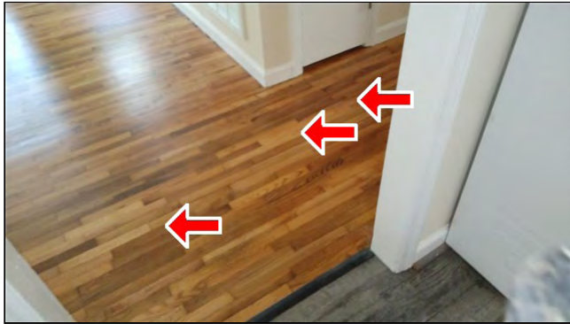
4.2 Item 1(Picture) Raised area in the flooring
