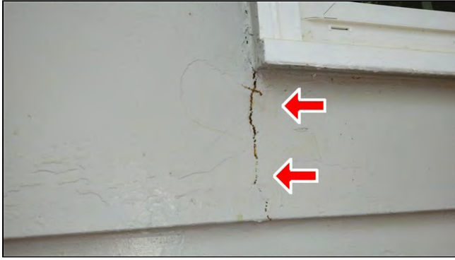
2.0 Item 3(Picture) Damaged siding noted
