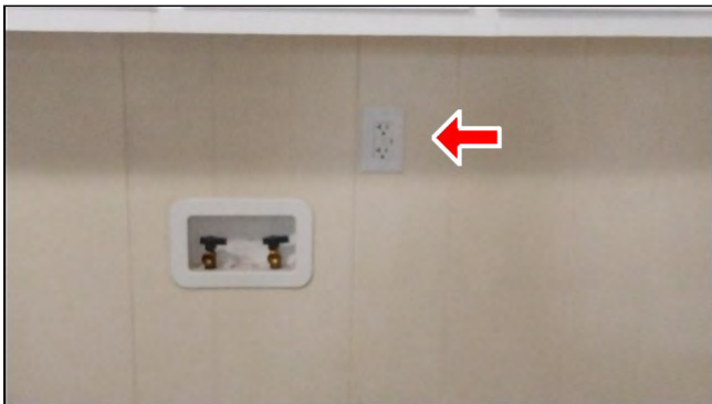
8.8 Item 1(Picture) The GFCI at the laundry areas is not functional
