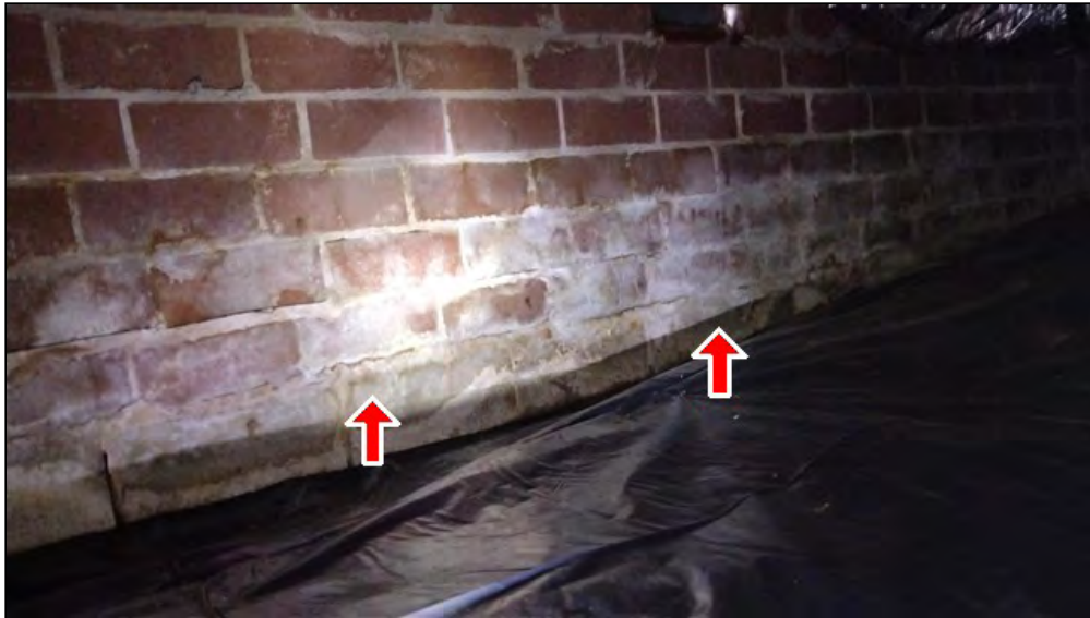
1.0 Item 9(Picture) Whited efflorescence on the foundation walls in the crawlspace
