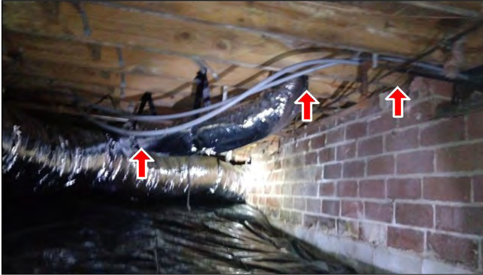
5.1 Item 2(Picture) Polybutylene piping noted
