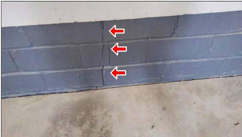
1.0 Item 8(Picture) Structural cracking noted in the homes foundation wall next to the carport concrete slab
