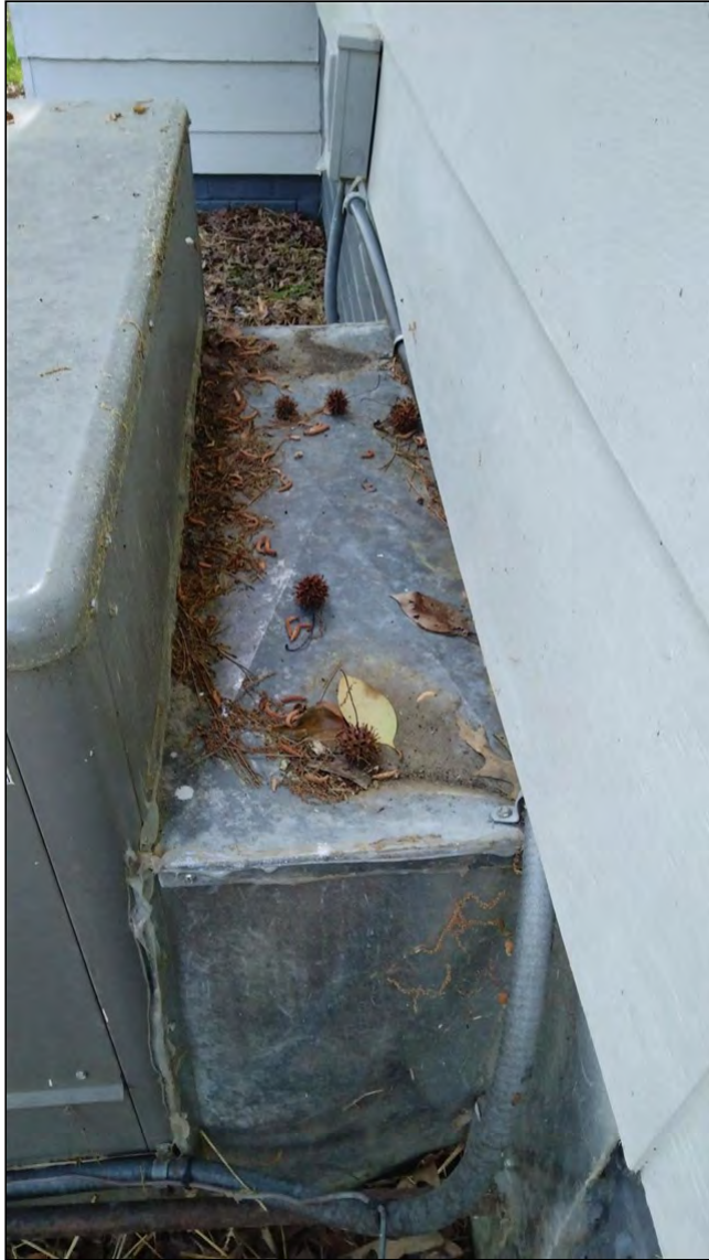
10.3 Item 1(Picture) Metal holding water and rusting
