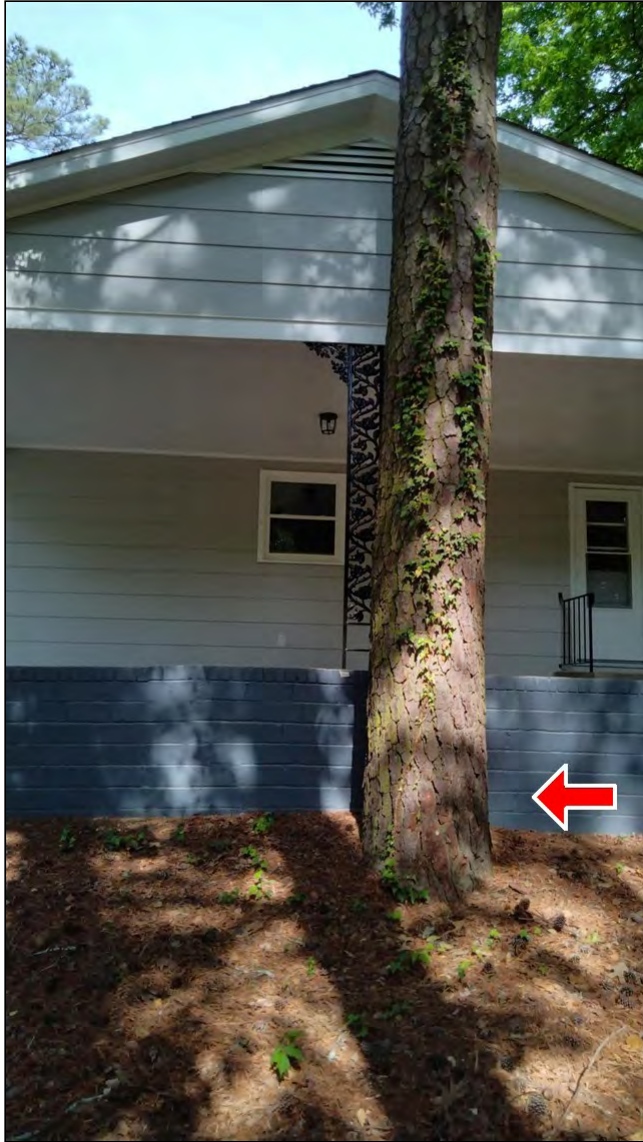
2.8 Item 1(Picture) A very large pine tree is growing against the foundation and the tree roots are causing damaged to the foundation
