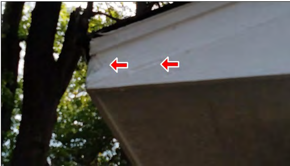
2.1 Item 3(Picture) Deterioration / damage noted
