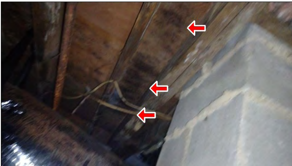
1.2 Item 9(Picture) Fungal growth with deterioration noted
