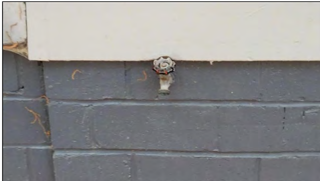
5.2 Item 1(Picture) Loose hose bib noted
