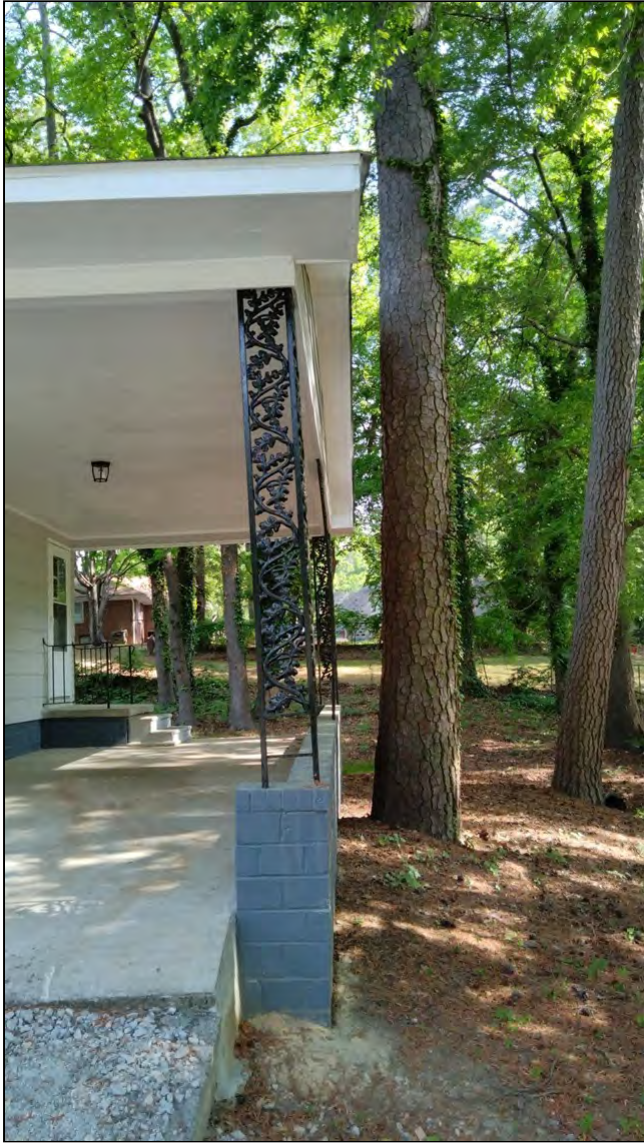
1.0 Item 12(Picture) Leaning foundation wall
