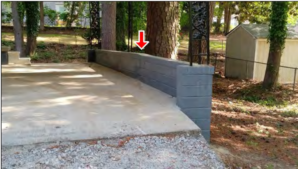
1.0 Item 10(Picture) Heaving foundation wall
