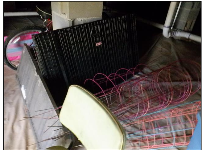
13.4 CRAWLSPACE DEBRIS/CELLULOSE (Picture 3)
