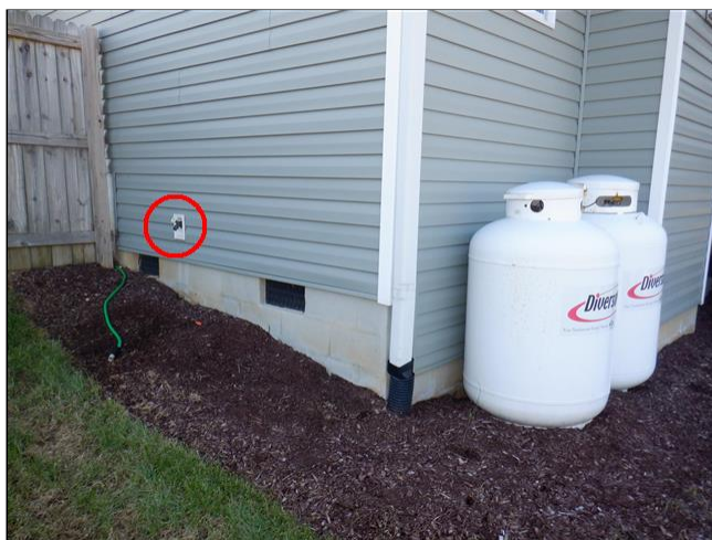
11.5 EXTERIOR FAUCET(S) (Picture 1)
