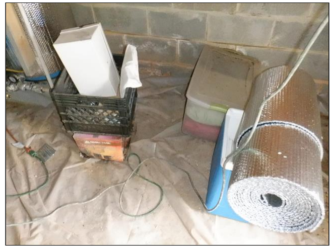
13.4 CRAWLSPACE DEBRIS/CELLULOSE (Picture 1)
