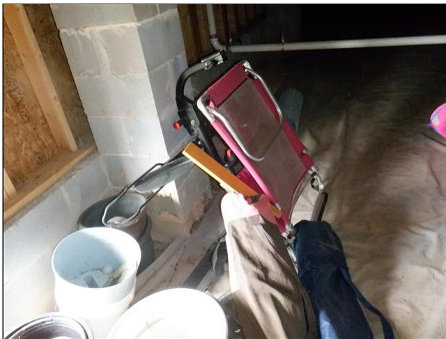
13.4 CRAWLSPACE DEBRIS/CELLULOSE (Picture 4)
