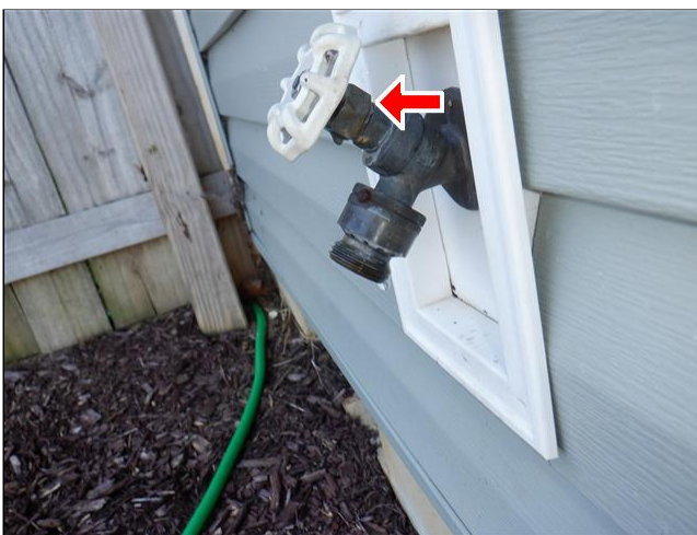
11.5 EXTERIOR FAUCET(S) (Picture 2)
