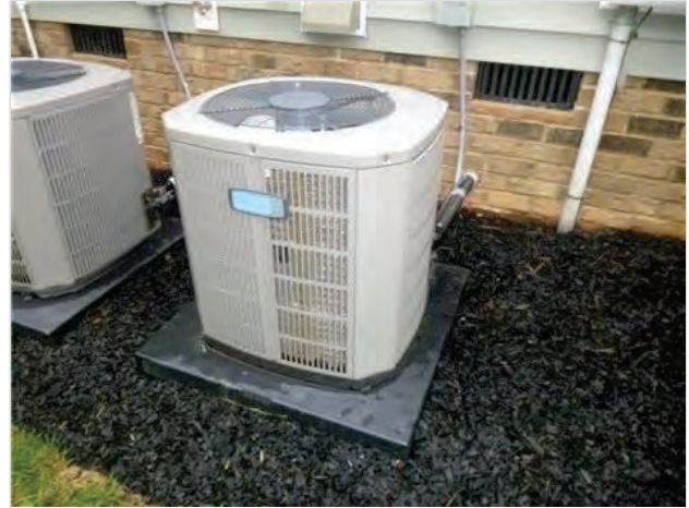
Upper Level HVAC Equipment
