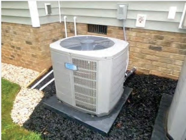
Lower Level HVAC Equipment
