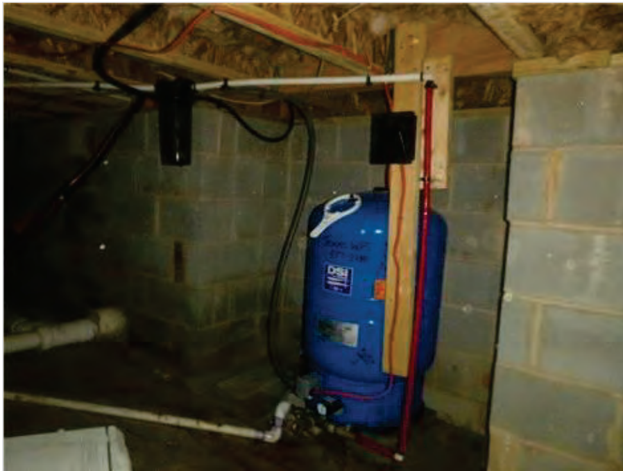
Pressure Tank In Crawl Space
