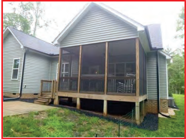
Missing Handrails at Rear Screened Porch Steps
