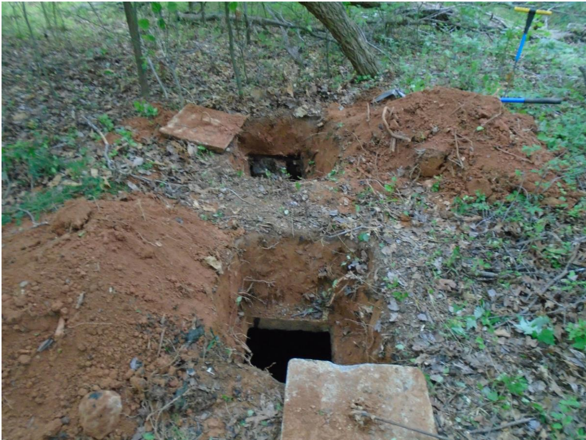
Septic Tank Location
