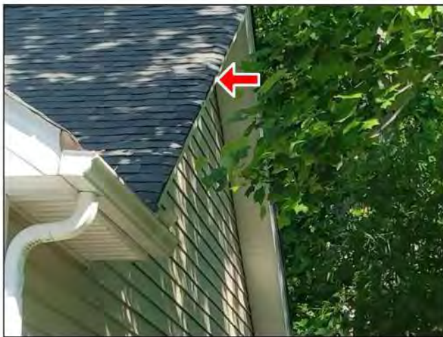
2.0 Item 5(Picture) Torn shingle notes
