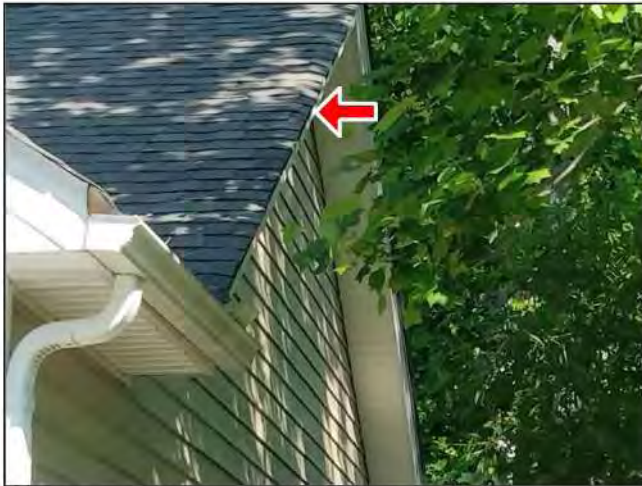
2.0 Item 5(Picture) Torn shingle notes
