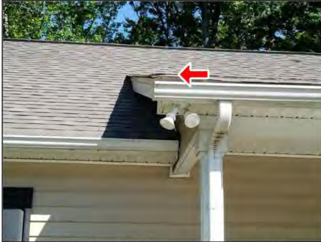
2.0 Item 6(Picture) Shingles are starting to bend
