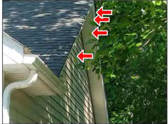
2.0 Item 7(Picture) Shingles are starting to bend
