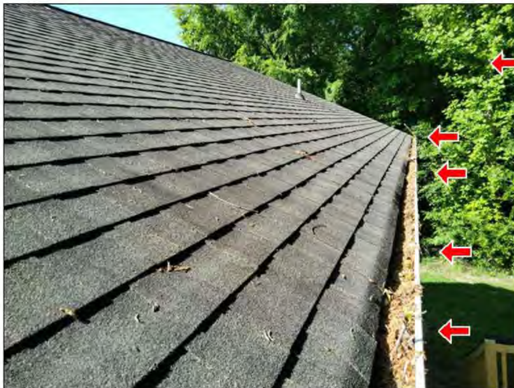
2.1 Item 2(Picture) Gutters are full of debris
