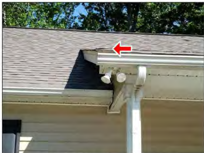
2.0 Item 6(Picture) Shingles are starting to bend
