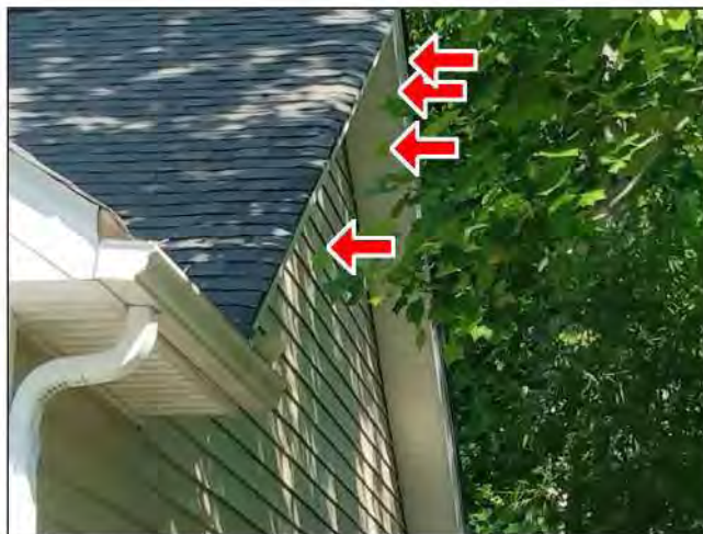
2.0 Item 7(Picture) Shingles are starting to bend
