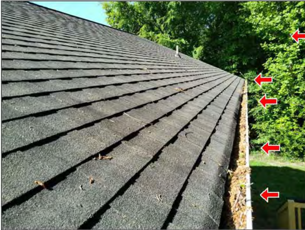
2.1 Item 2(Picture) Gutters are full of debris
