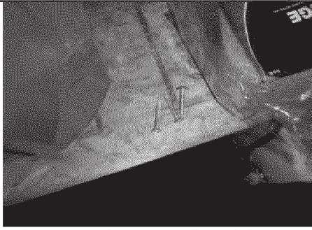
Improper Screws at Panel Cover
