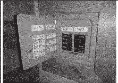
Upper Sub Panel
