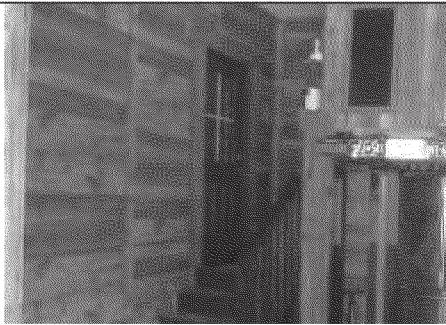
Non Fire-Rated Garage Service Door
