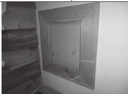
Inaccessible Electric Panel
