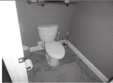
Loose Toilet in Master Bathroom
