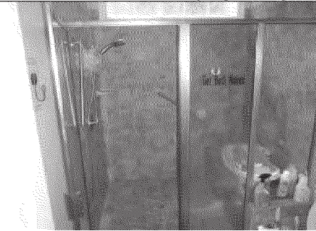
Hot/Cold Supply Lines Reversed
