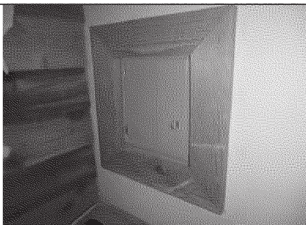
Inaccessible Electric Panel
