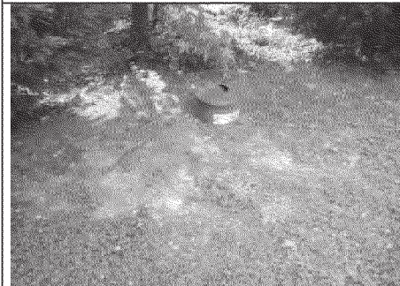
Underground Propane Tank
