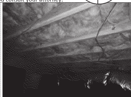
Suspect Mold at Framing
