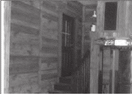
Non Fire-Rated Garage Service Door
