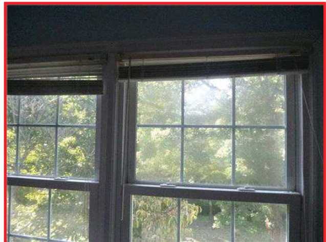
Failed Thermal Seal Window
