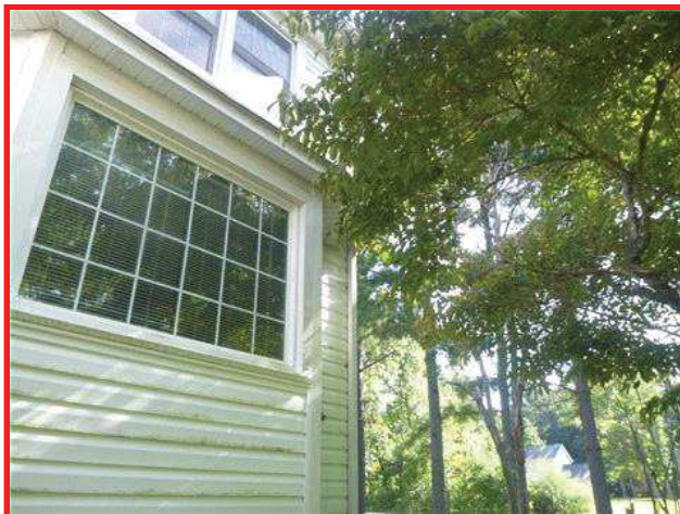
Tree in Contact with Roof
