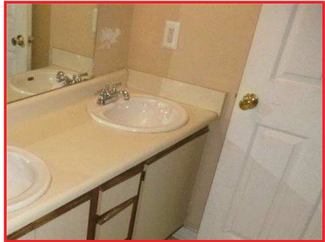
GFI Outlet Wired to Laundry Breaker
