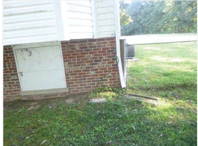
Copper Propane Lines
