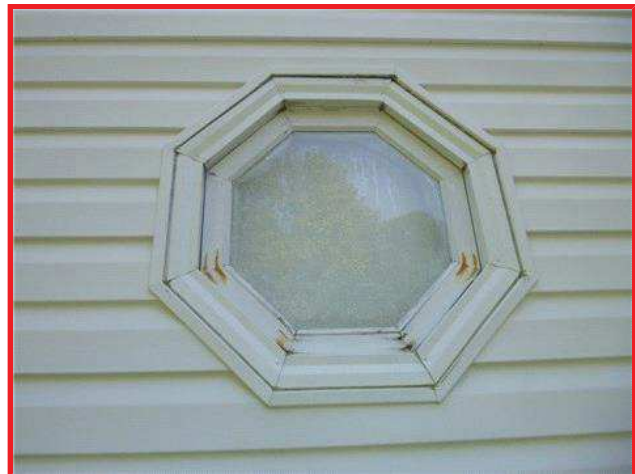
Deteriorated Trim at Octagon Window
