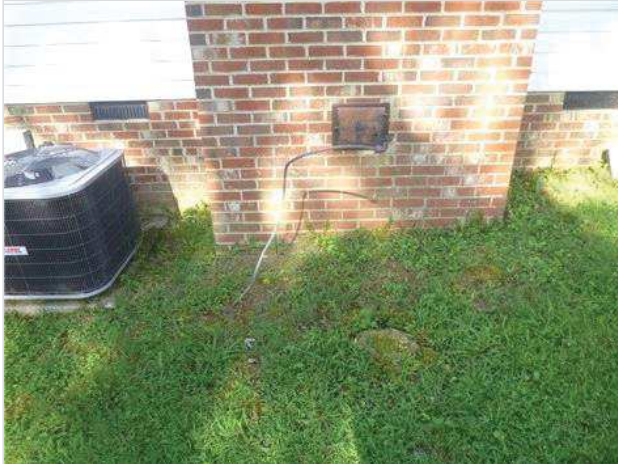
Copper Propane Lines
