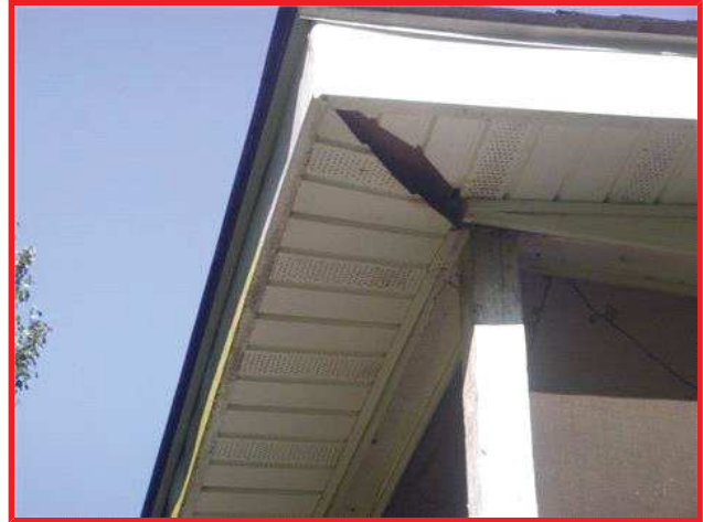
Loose Soffit at Porch
