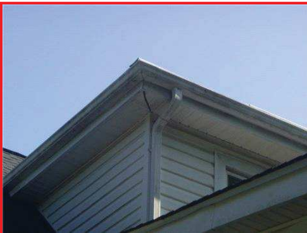
Loose Upper Soffit
