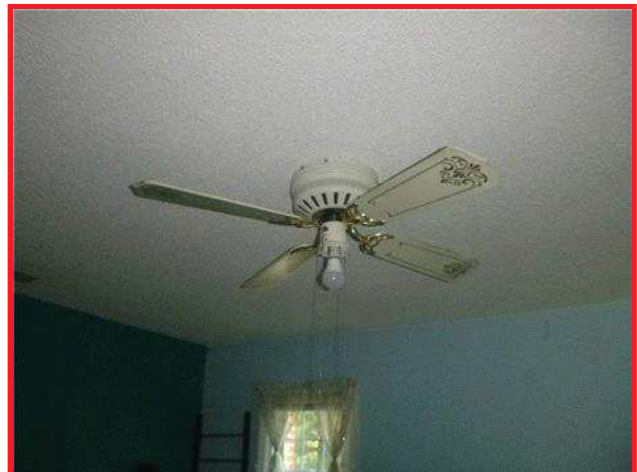
Missing Globe at Ceiling Fan Light Fixture
