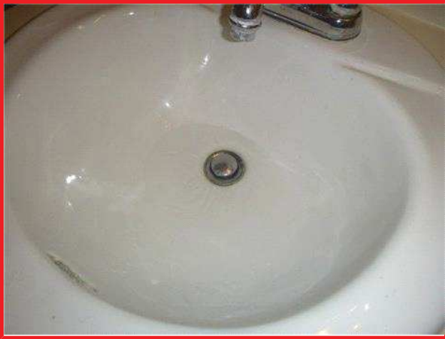
Master Bathroom Sink Drains Slowly
