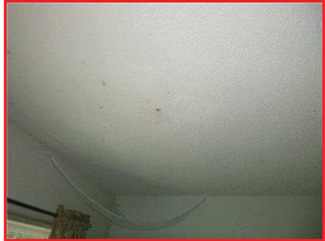
Moisture Damaged Bedroom Ceiling / Suspect Asbestos
