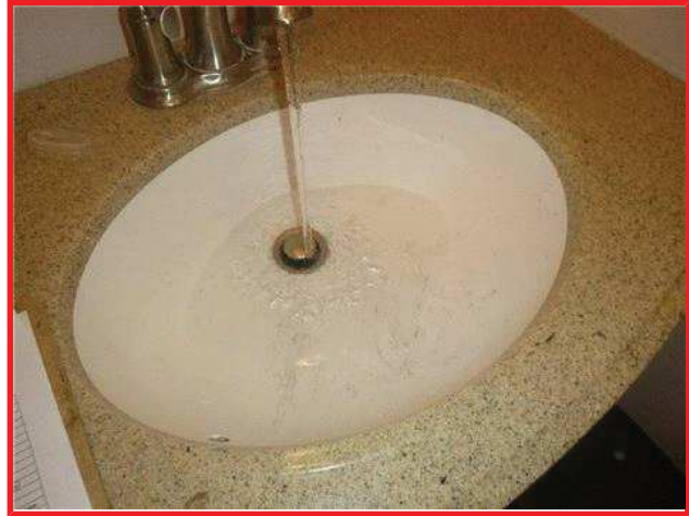
Bathroom Sink Drains Slowly
