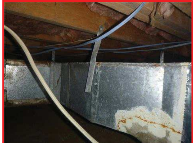
Improperly Supported Plenum
