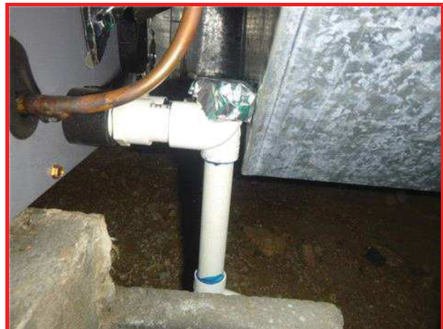
Improper / Capped Secondary Condensate Drain Line
