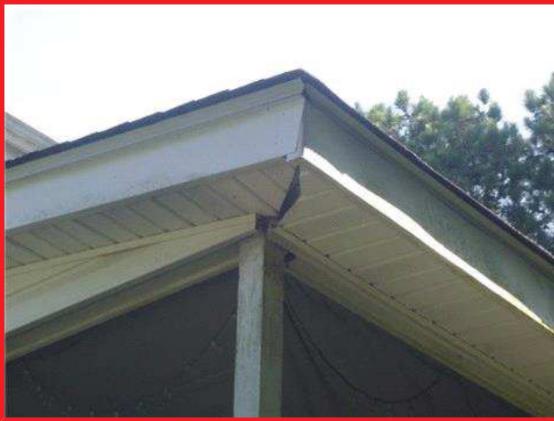
Loose Soffit at Porch
