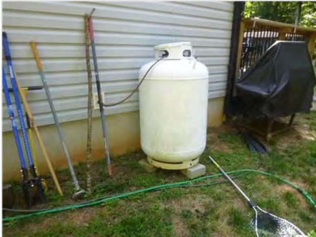
Above Ground Propane Tank
