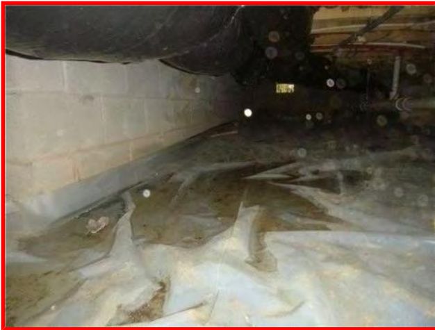
Pooling Water in Crawl Space
