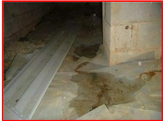
Pooling Water in Crawl Space
