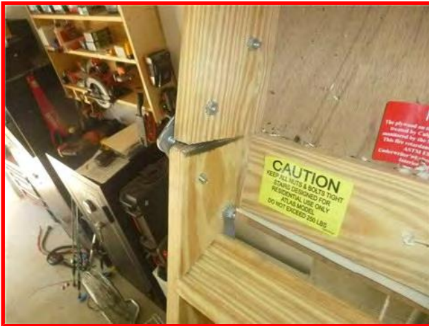
Missing Hardware at Attic Access Ladder
