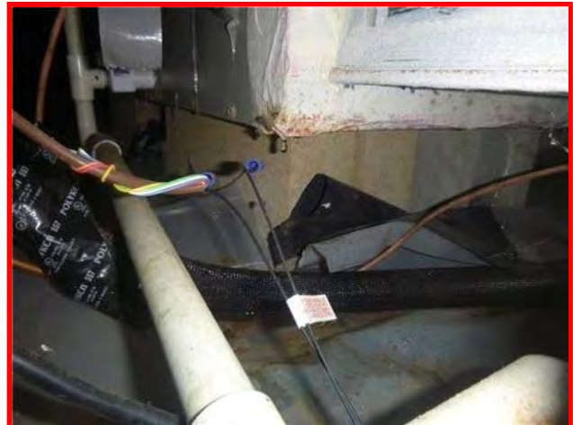
Leak at Heat Pump Condensate Line
