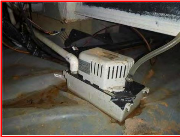
Standing Water at Condensate Pump
