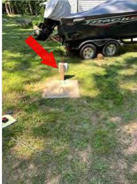
Control Panel Not 12" Above Ground
