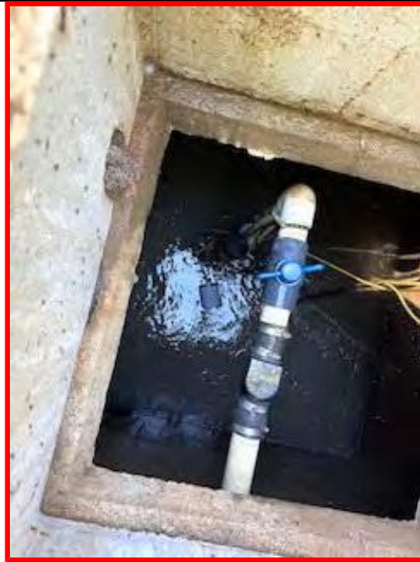
Pump Tank Riser At Grade
