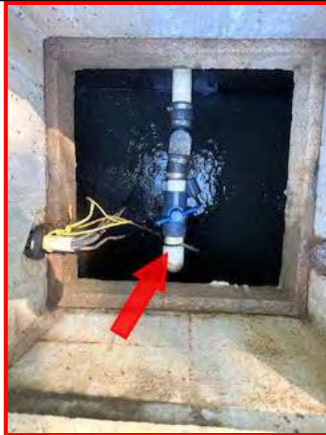
Leak At Check Valve At Pump Tank Riser
