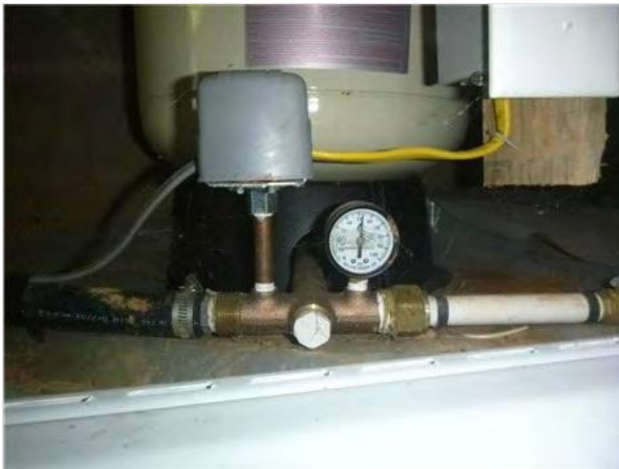
Well Gauges And Controls
