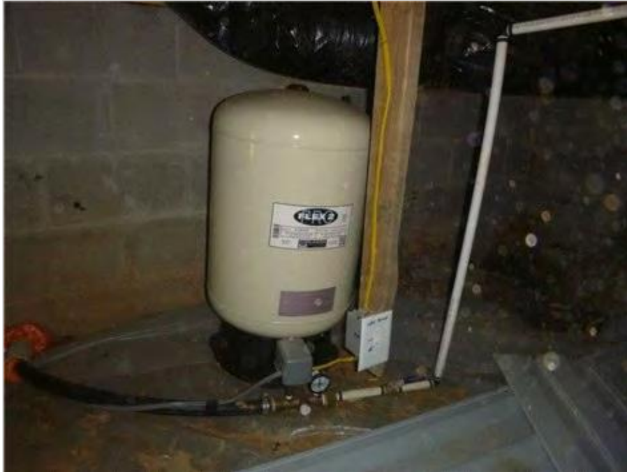
Pressure Tank In rawl Space
