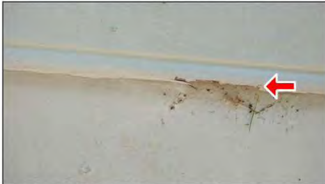
2.0 Item 2(Picture) Deteriorated siding
