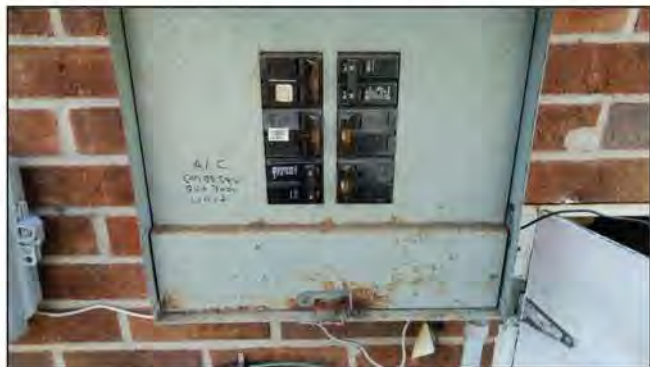
8.3 Item 1(Picture) Breakers are not labeled
