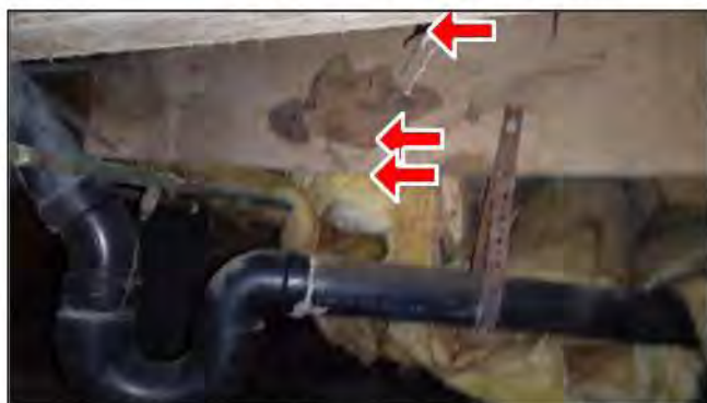
1.2 Item 1(Picture) Broken floor joist at a knot in the wood
