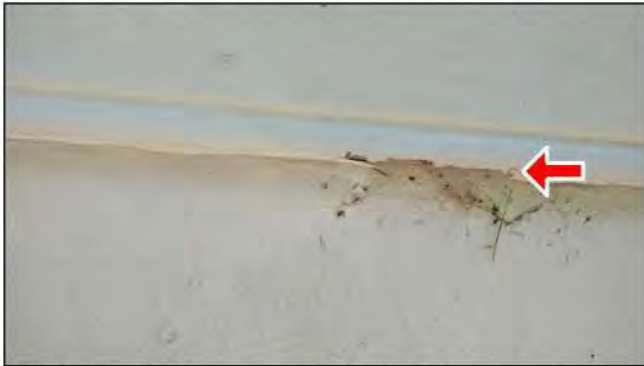
2.0 Item 2(Picture) Deteriorated siding
