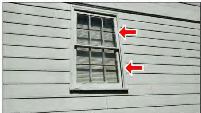
2.3 Item 4(Picture) Missing storm window
