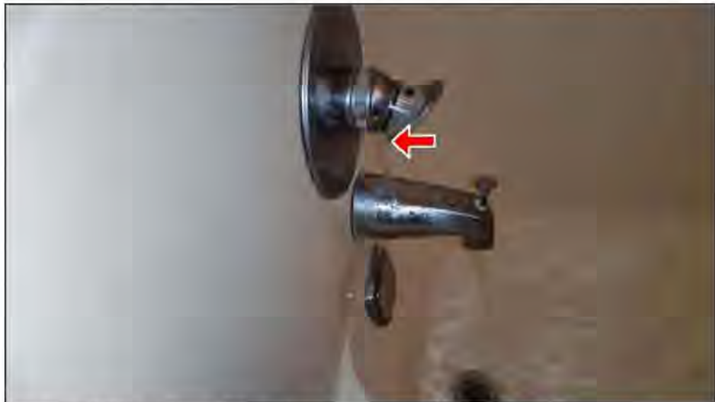
7.2 Item 2(Picture) Leak noted at he shower faucer handle
