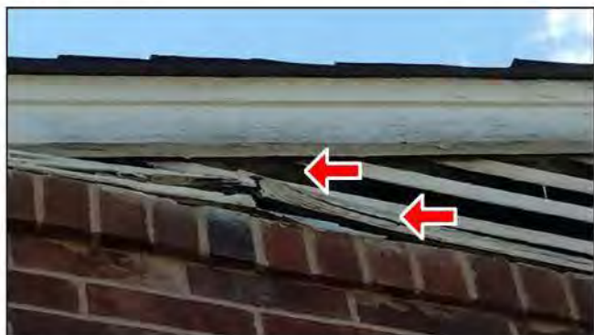
2.0 Item 6(Picture) Deterioration noted at the gable vent
