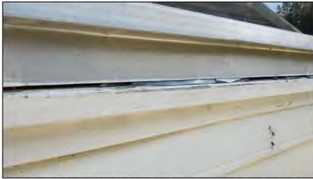
2.4 Item 1(Picture) Broken storm window glass
