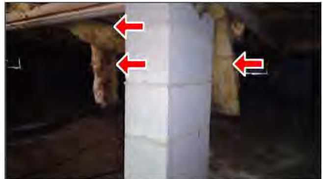
11.1 Item 2(Picture) The flooring insulation has fallen in areas of the crawlspace
