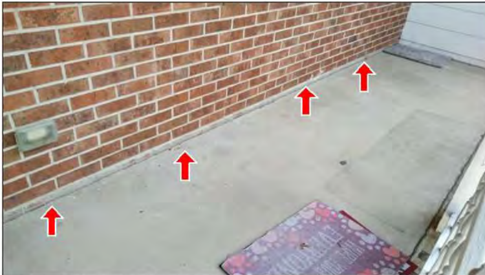
2.5 Item 5(Picture) Settled front porch
