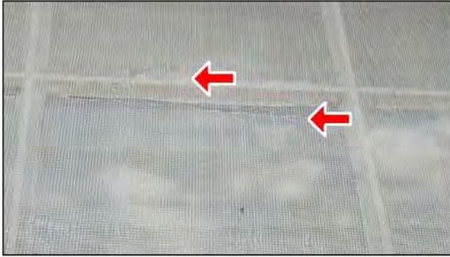
2.3 Item 5(Picture) Torn screens
