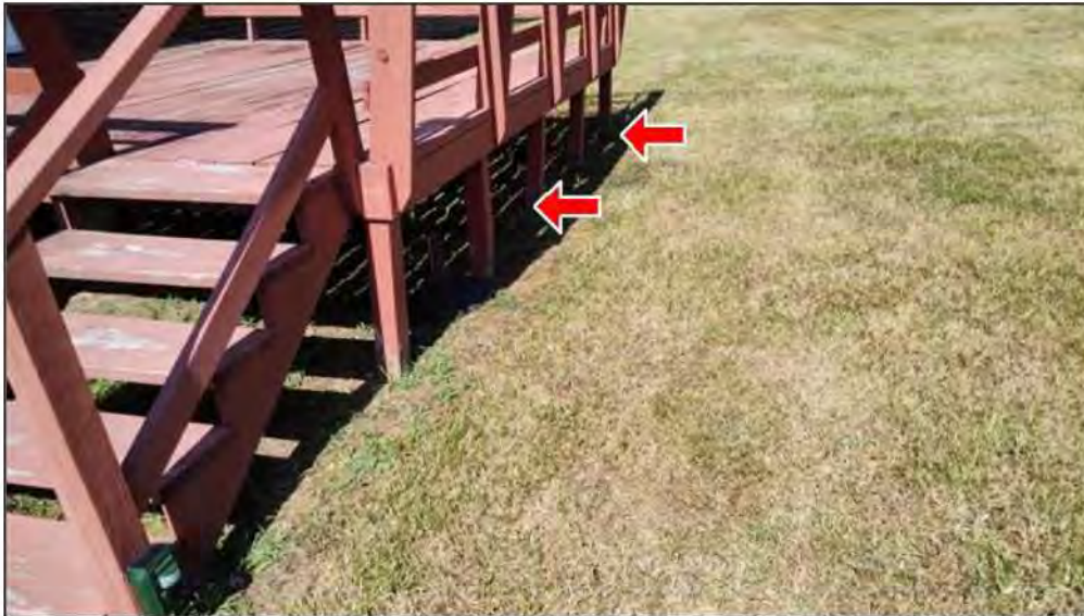
2.8 Item 2(Picture) Post need braces as they are starting to lean
