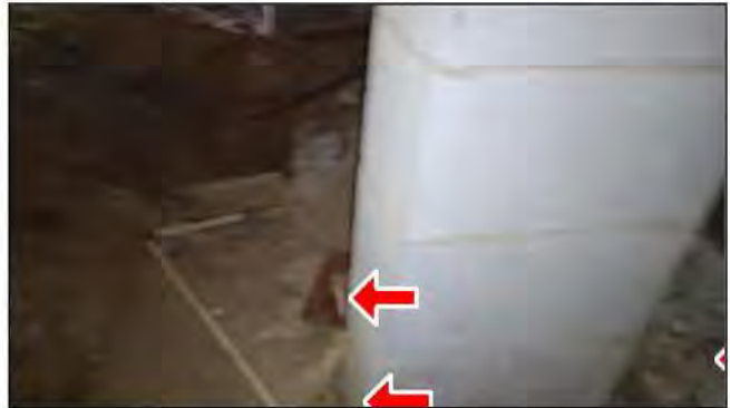
1.1 Item 2(Picture) Footers have not been back filled
