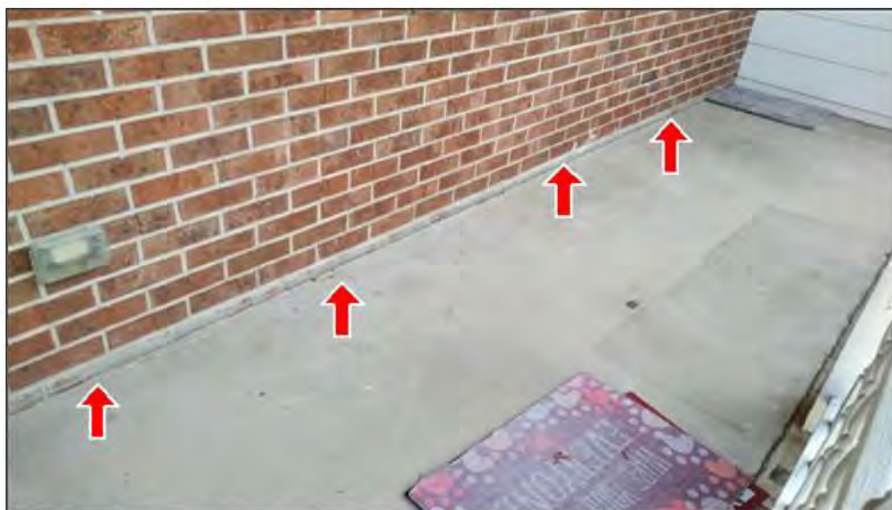
2.5 Item 5(Picture) Settled front porch
