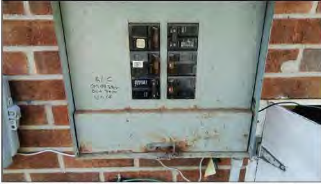
8.3 Item 1(Picture) Breakers are not labeled
