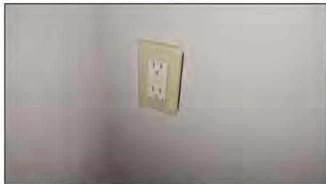
8.9 Item 1(Picture) GFCI's not resetting
