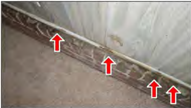
4.7 Item 3(Picture) Moisture stains noted
