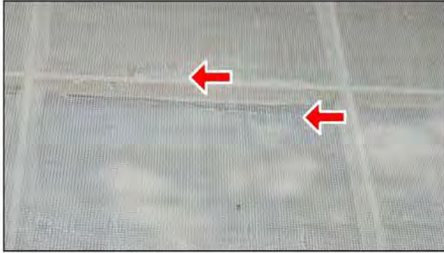
2.3 Item 5(Picture) Torn screens
