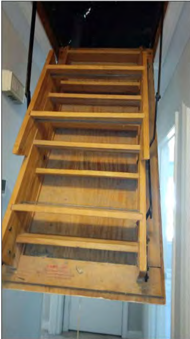
1.7 Item 1(Picture) Door missing insulation and weather stripping
