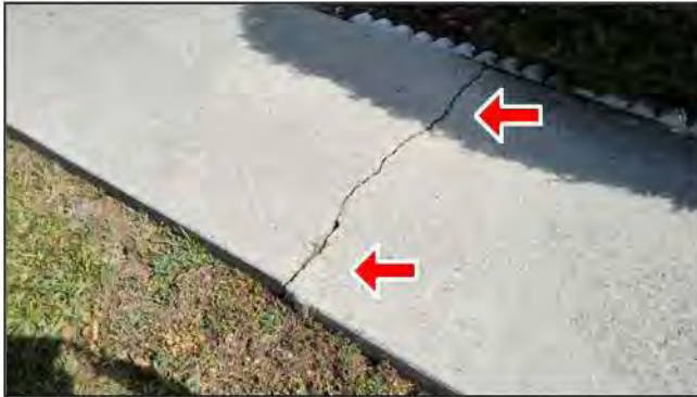
2.7 Item 4(Picture) Cracking with raised areas noted
