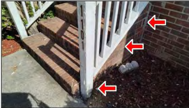
2.2 Item 1(Picture) Failing paint on the front porch railing
