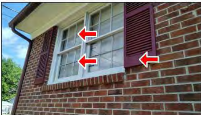
2.3 Item 3(Picture) Missing screens and glass
