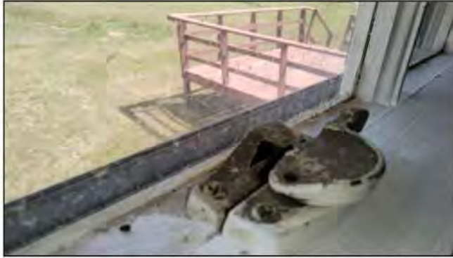
4.6 Item 1(Picture) Window latches are not aligning
