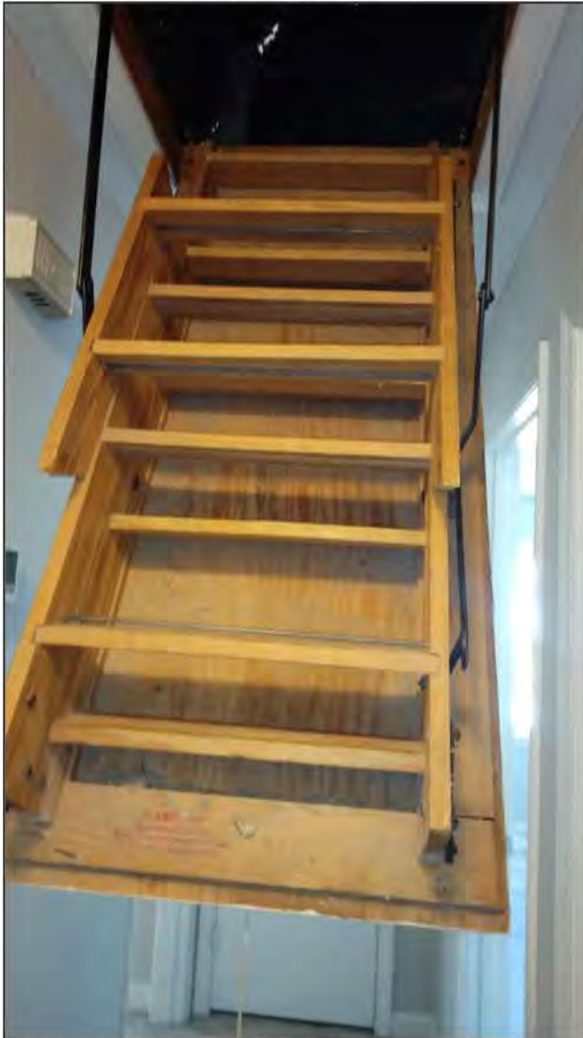
1.7 Item 1(Picture) Door missing insulation and weather stripping
