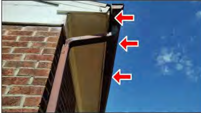
3.1 Item 2(Picture) Loose gutters noted on the home
