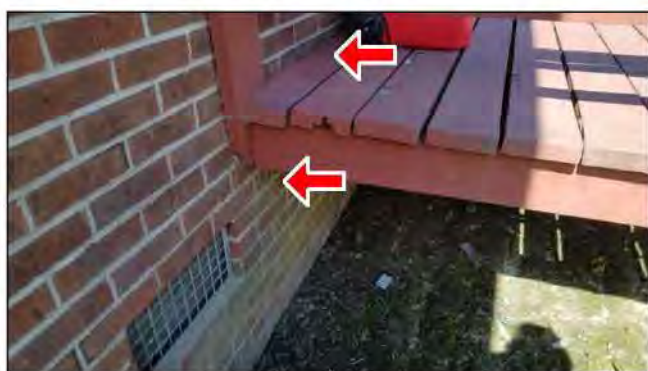
2.8 Item 3(Picture) No flashings installed
