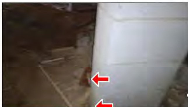
1.1 Item 2(Picture) Footers have not been back filled
