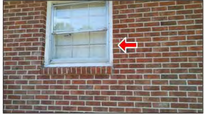
2.3 Item 6(Picture) missing screen
