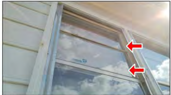
2.4 Item 2(Picture) broken glass
