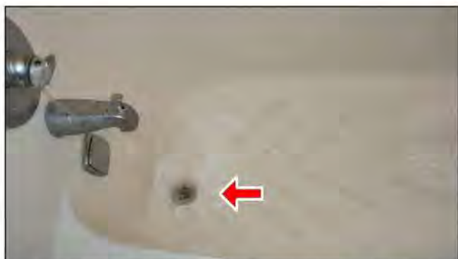
7.2 Item 1(Picture) Tub stopper missing
