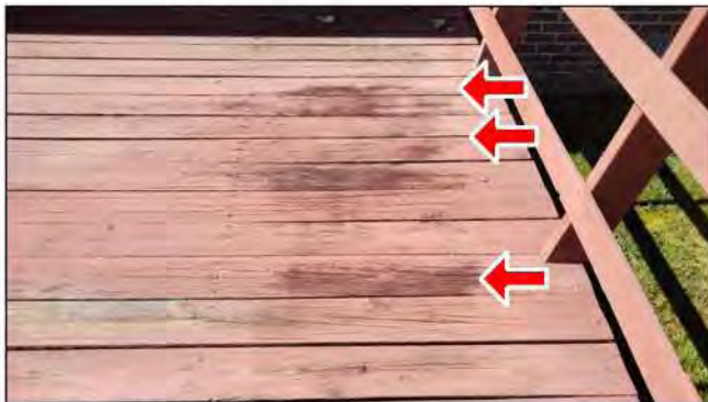
2.8 Item 9(Picture) Deteriorated decking boards
