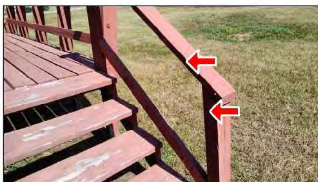
2.8 Item 4(Picture) Loose hand rail
