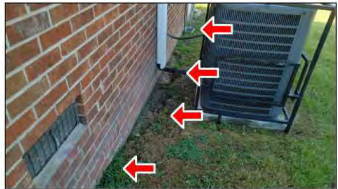
2.10 Item 2(Picture) Erosion along the foundation
