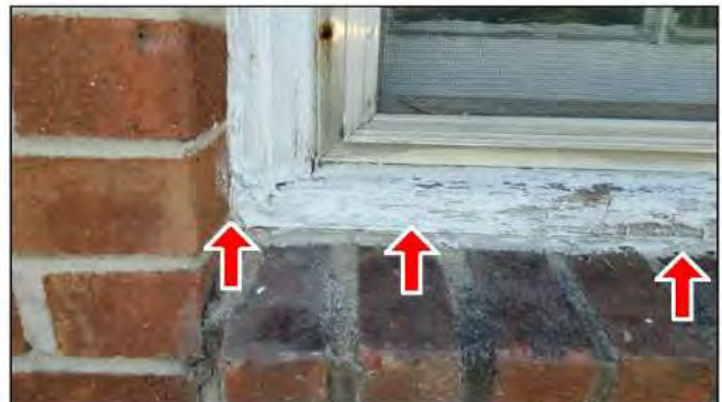
2.2 Item 4(Picture) Failing paint and caulk at the windows
