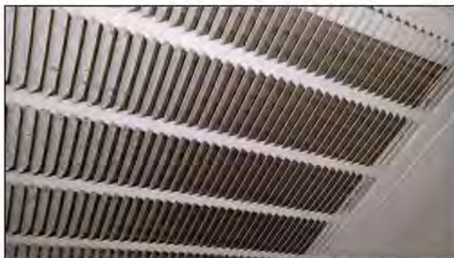
10.6 Item 1(Picture) Clogged filters noted
