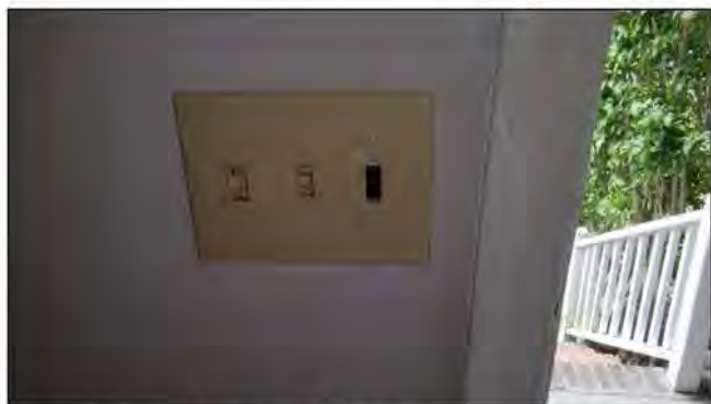
8.7 Item 1(Picture) Switch missing leaving exposed wiring
