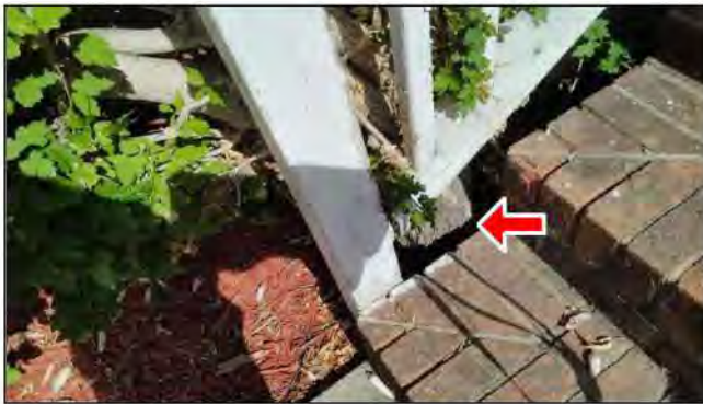
2.7 Item 5(Picture) Tree root growing against and under the front steps
