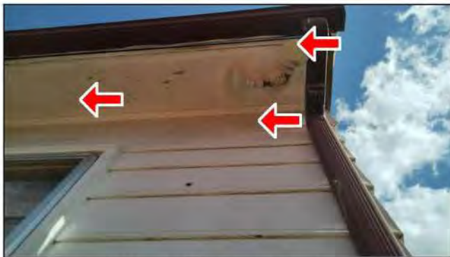
2.2 Item 10(Picture) Failing paint noted
