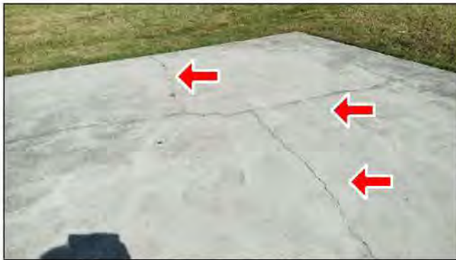
2.7 Item 1(Picture) Common cracks noted in the driveway
