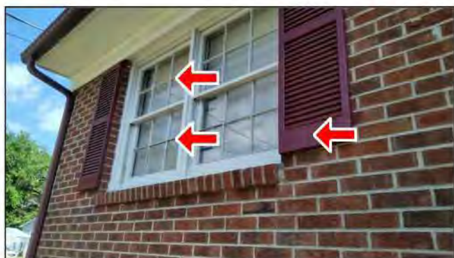
2.3 Item 3(Picture) Missing screens and glass
