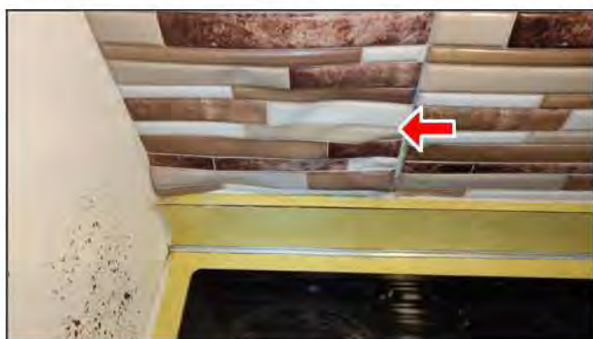
4.1 Item 2(Picture) Stick on tile are loose
