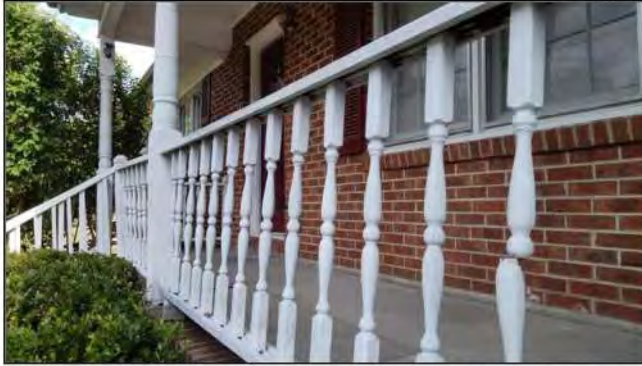
2.5 Item 1(Picture) Loose deteriorated rails and pickets
