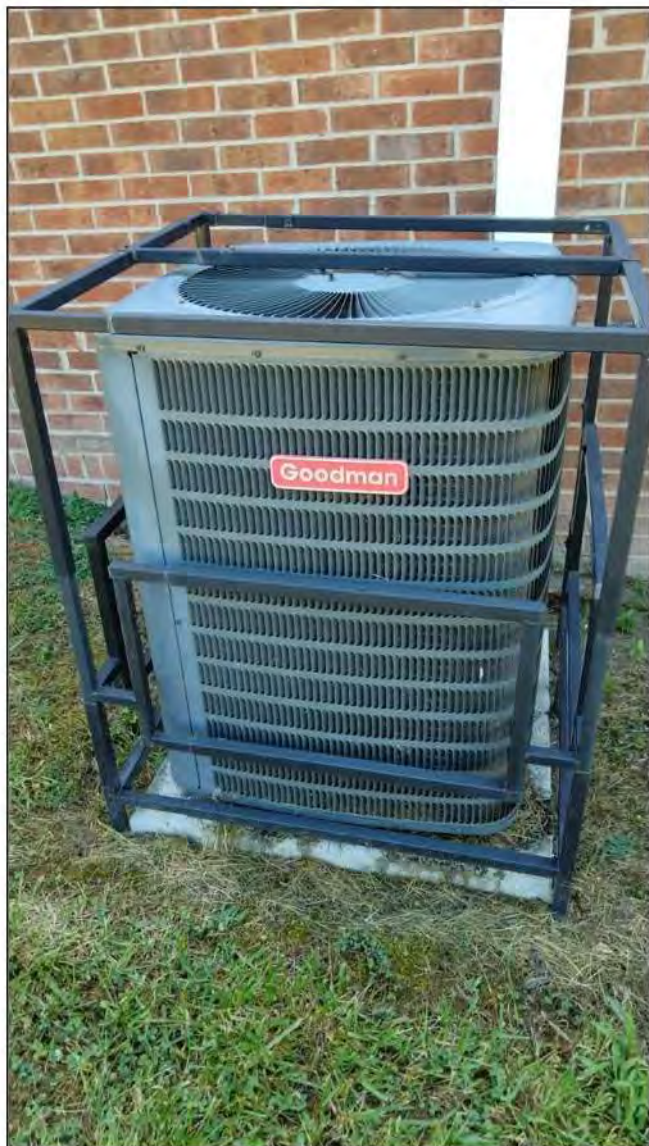
9.0 Item 1(Picture) The AC condenser unit
