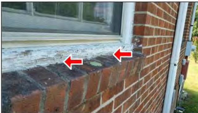
2.2 Item 5(Picture) Failing paint at the windows
