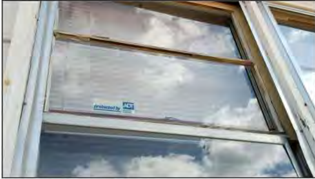
2.3 Item 1(Picture) Failing and missing glazing
