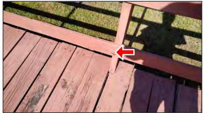
2.8 Item 8(Picture) Cracking boards noted
