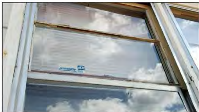
2.3 Item 1(Picture) Failing and missing glazing
