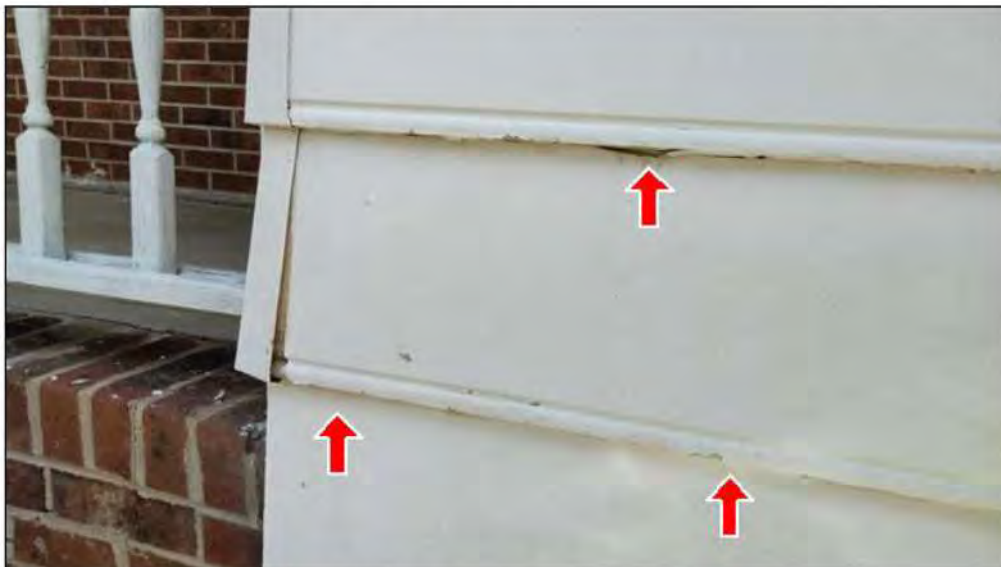
2.0 Item 3(Picture) Damaged siding
