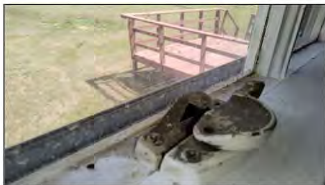
4.6 Item 1(Picture) Window latches are not aligning
