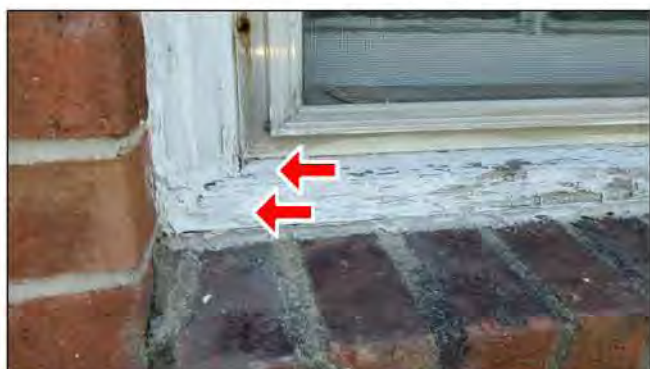
2.3 Item 2(Picture) Deterioration noted
