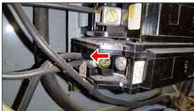
8.5 Item 2(Picture) Double tapped breakers noted
