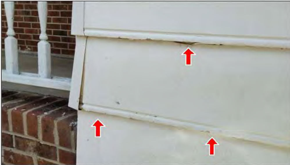
2.0 Item 3(Picture) Damaged siding
