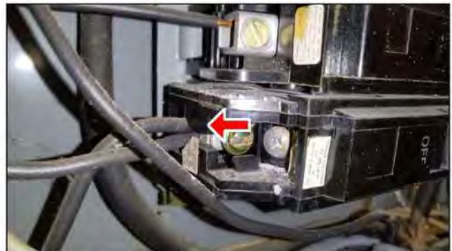
8.5 Item 2(Picture) Double tapped breakers noted
