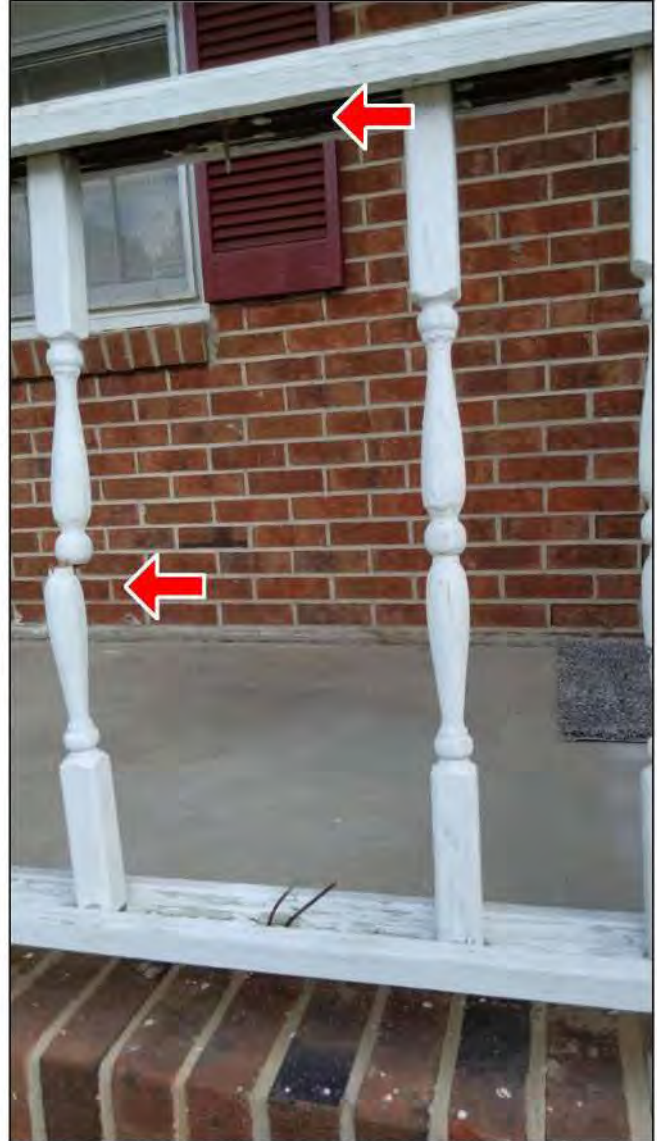
2.5 Item 2(Picture) broken and missing pickets
