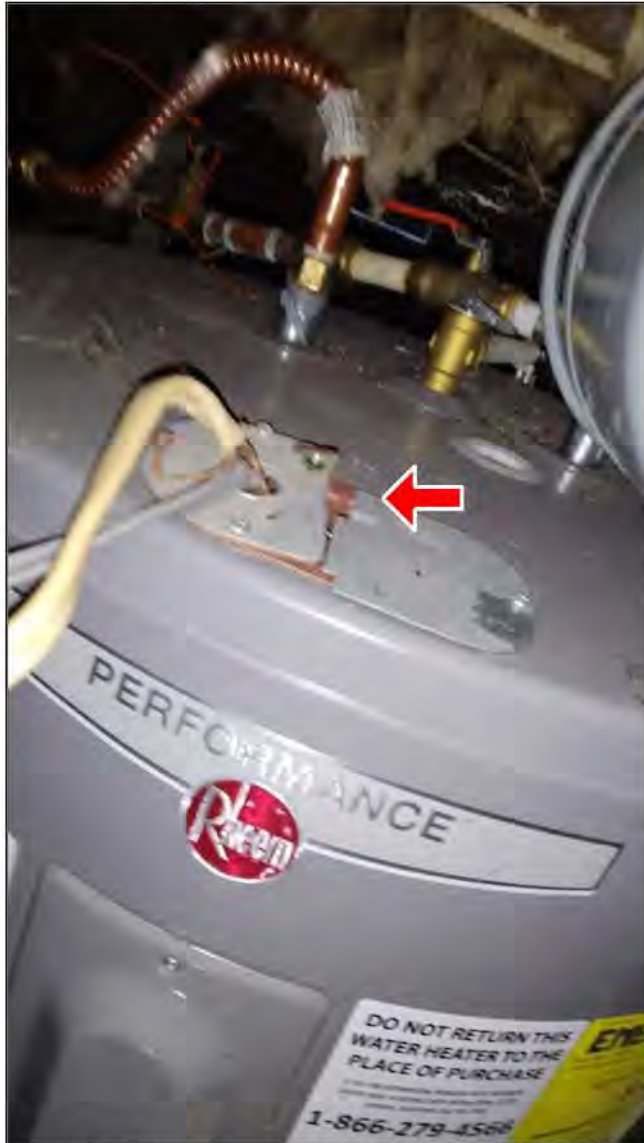
6.3 Item 1(Picture) Wiring not properly connected
