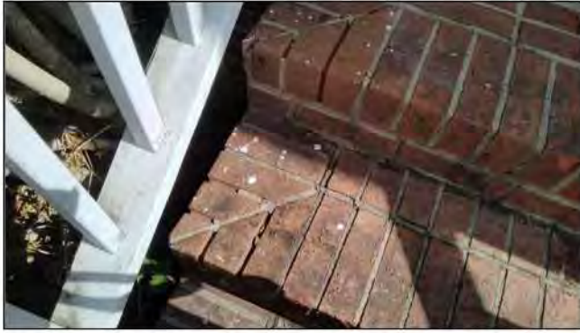
2.6 Item 1(Picture) missing mortar noted
