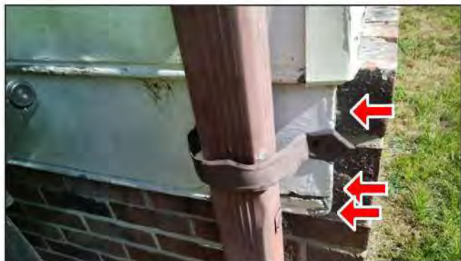
2.0 Item 4(Picture) Deteriorated siding in the lower areas.
