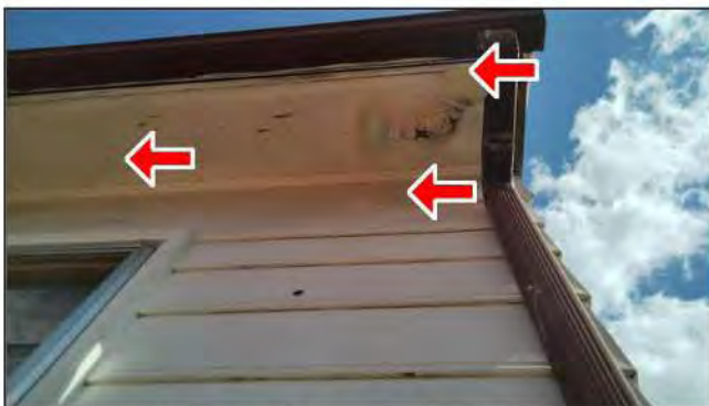
2.2 Item 10(Picture) Failing paint noted
