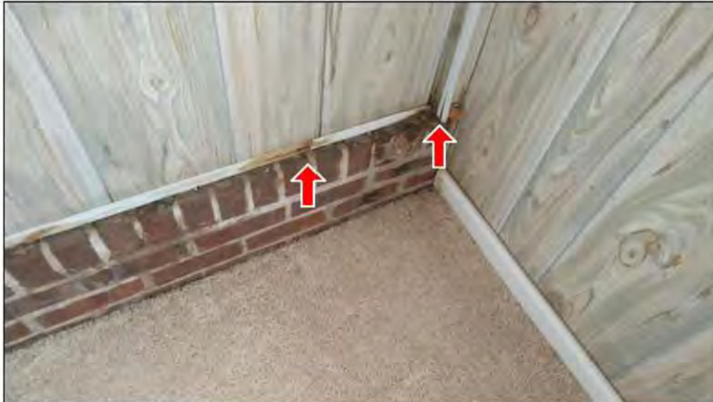
4.7 Item 1(Picture) moisture stains and damage indicate later water leaking into the home in these areas
