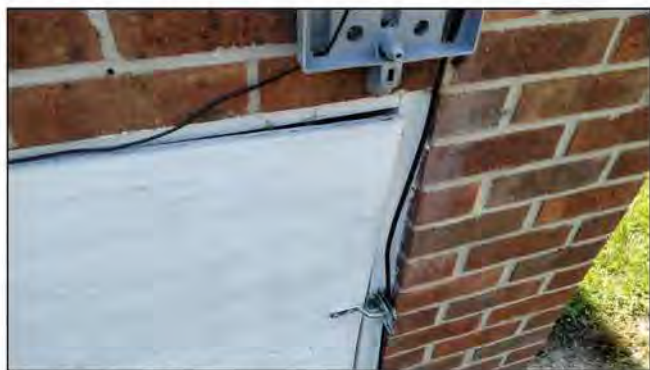
1.3 Item 2(Picture) Gaps at the crawlspace door
