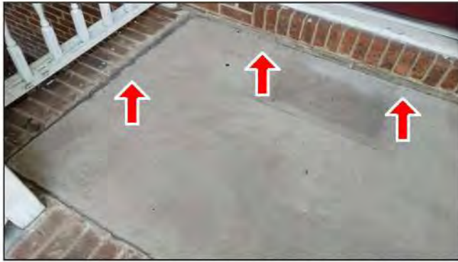
2.5 Item 4(Picture) Front porch has settled and is sloped towards the home
