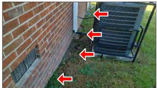
2.10 Item 2(Picture) Erosion along the foundation
