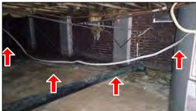
8.6 Item 1(Picture) Wiring not secured in the crawlspace
