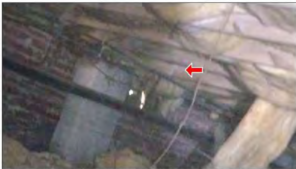
1.2 Item 3(Picture) Sistered floor framing not supported on the ends
