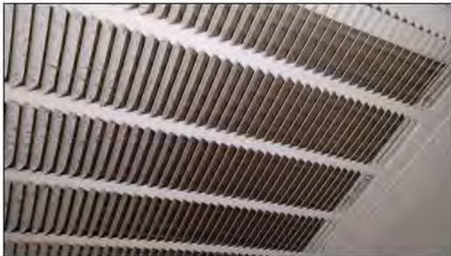
10.6 Item 1(Picture) Clogged filters noted
