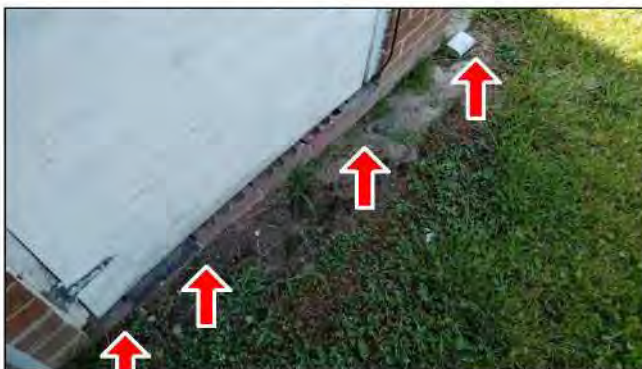
2.10 Item 1(Picture) Erosion along the foundation
