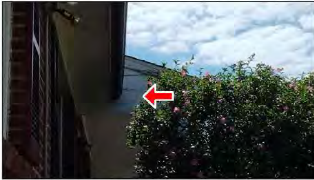
3.3 Item 1(Picture) Missing kickout flashings with deteriorated siding
