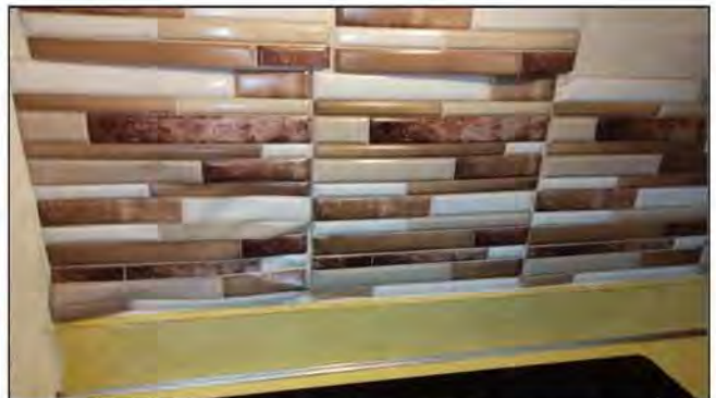
4.1 Item 3(Picture) Stick on tile are loose
