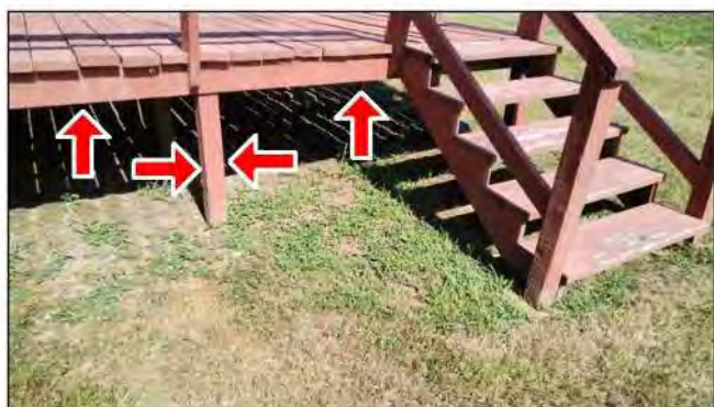
2.8 Item 1(Picture) Missing 45% angle braces
