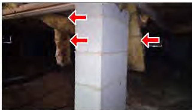
11.1 Item 2(Picture) The flooring insulation has fallen in areas of the crawlspace
