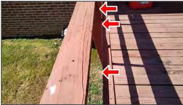
2.8 Item 7(Picture) Splintering hand rails
