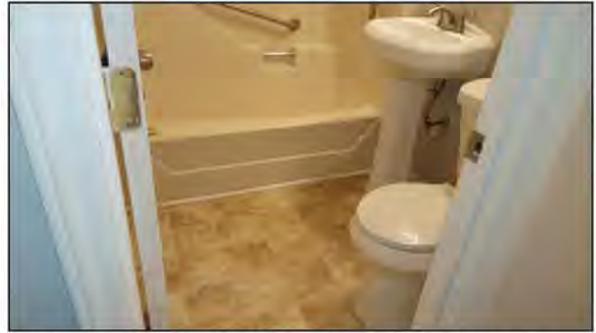
4.2 Item 3(Picture) Dip in the hall bathroom floor
