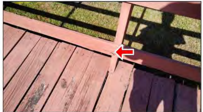
2.8 Item 8(Picture) Cracking boards noted
