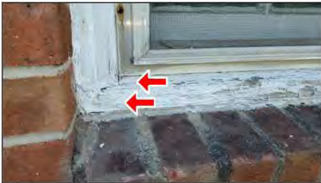
2.3 Item 2(Picture) Deterioration noted
