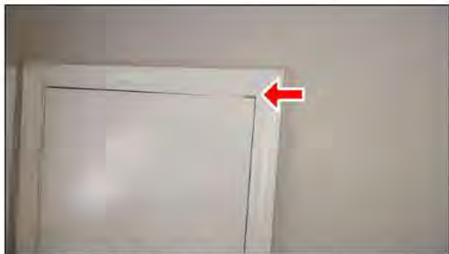
4.5 Item 1(Picture) Door will not open
