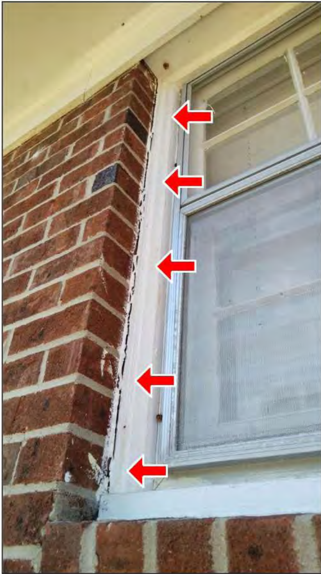
2.2 Item 8(Picture) Caulk has failed
