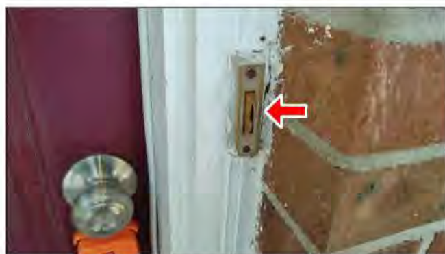
8.11 Item 1(Picture) Broken door bell cover
