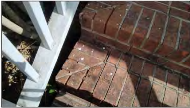
2.6 Item 1(Picture) missing mortar noted
