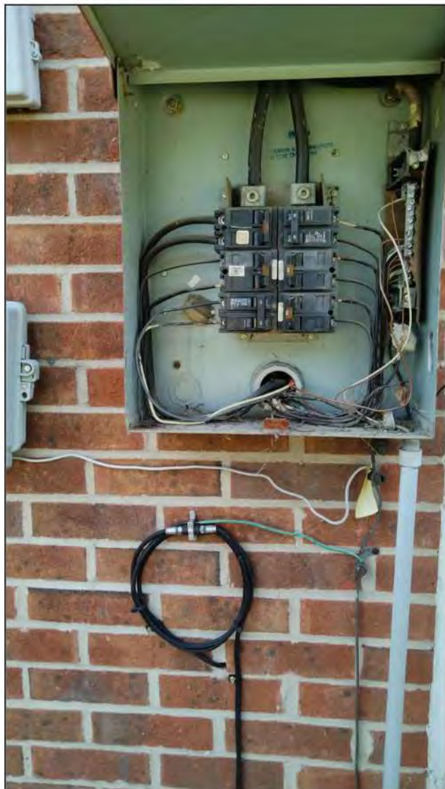
8.2 Item 1(Picture) The inside of the main electrical box
