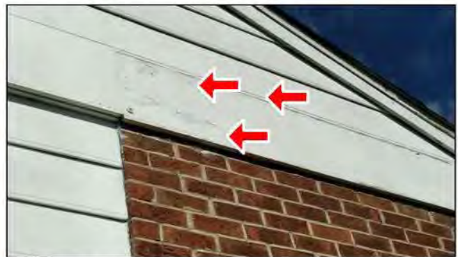
2.1 Item 3(Picture) Deterioration noted in the trim boards
