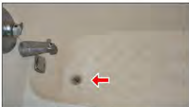
7.2 Item 1(Picture) Tub stopper missing
