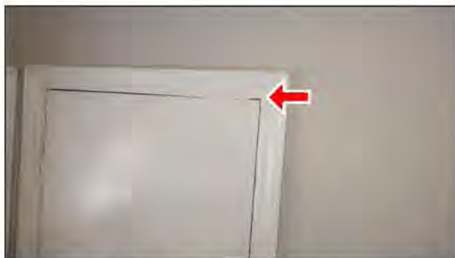
4.5 Item 1(Picture) Door will not open
