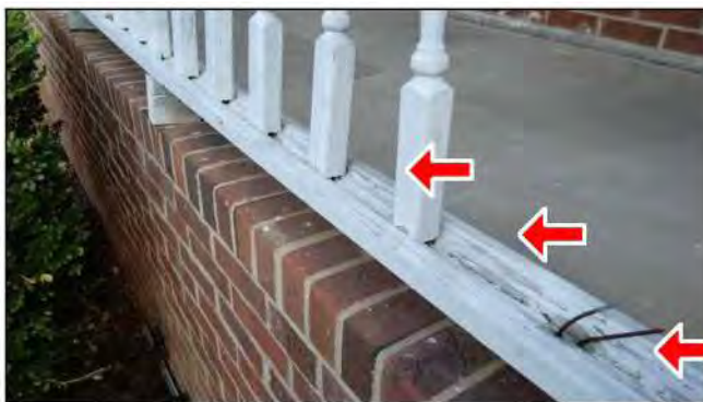
2.5 Item 3(Picture) Deteriorated railing and pickets
