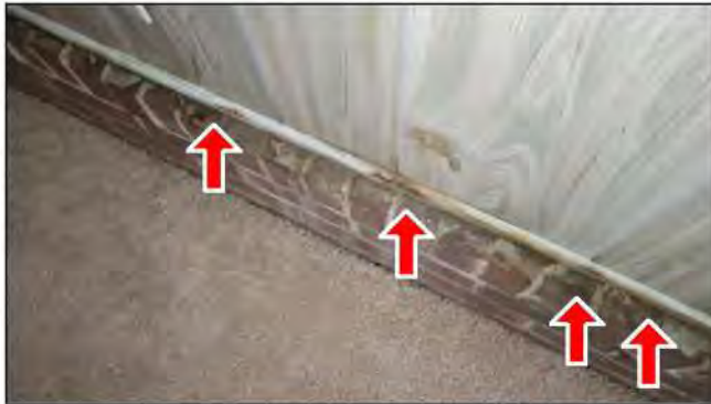
4.7 Item 3(Picture) Moisture stains noted
