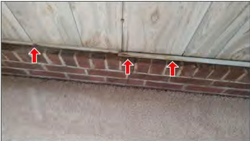
4.7 Item 2(Picture) Moisture stains noted
