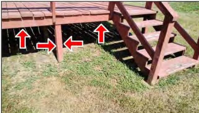
2.8 Item 1(Picture) Missing 45% angle braces
