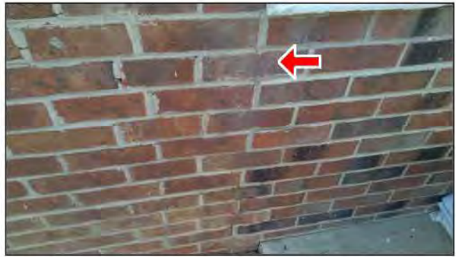
1.0 Item 2(Picture) Structural cracks in brickwork with cracked bricks noted
