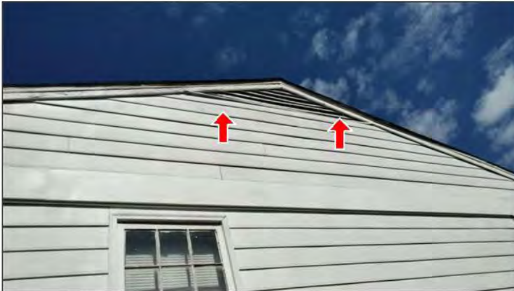
2.2 Item 6(Picture) Failing paint on the gable vents
