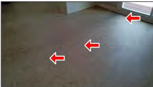
1.2 Item 4(Picture) Large dip in the kitchen floor
