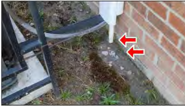
9.5 Item 1(Picture) The condensation tube is draining against the foundation
