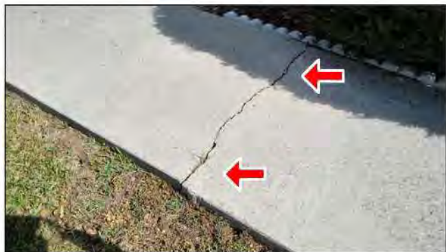
2.7 Item 4(Picture) Cracking with raised areas noted
