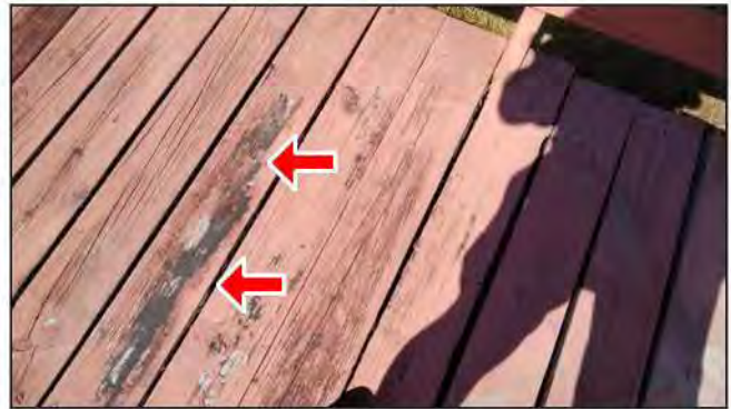
2.8 Item 10(Picture) Deteriorated deck boards
