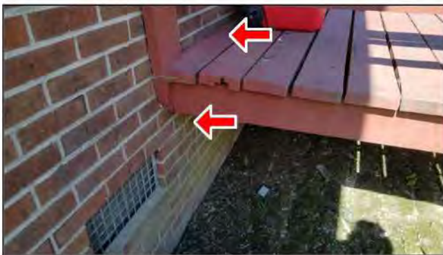
2.8 Item 3(Picture) No flashings installed
