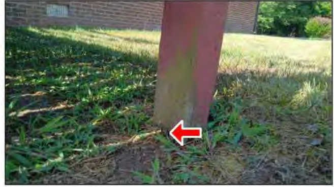
2.8 Item 12(Picture) Deterioration noted at grade
