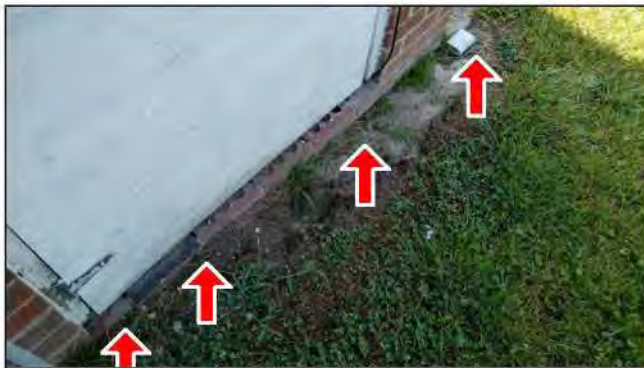
2.10 Item 1(Picture) Erosion along the foundation
