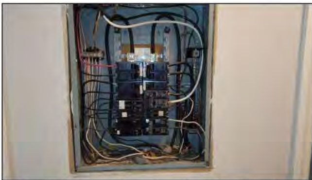
8.4 Item 1(Picture) The inside of the distribution panel box
