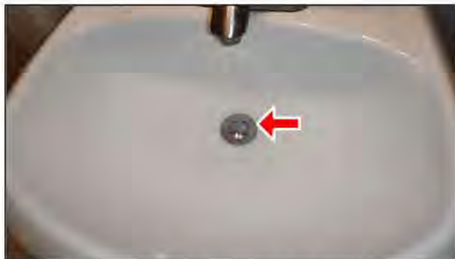
7.1 Item 1(Picture) Damaged sink stopper not functional
