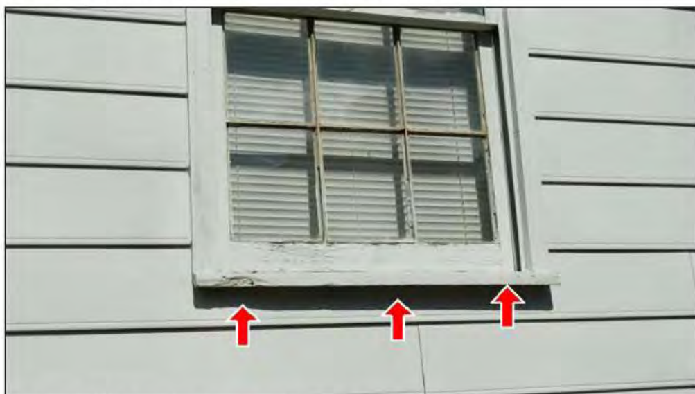
2.2 Item 7(Picture) Failing paint on the windows
