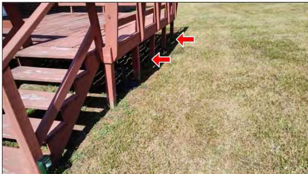
2.8 Item 2(Picture) Post need braces as thy are starting to lean
