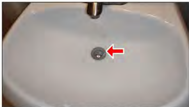
7.1 Item 1(Picture) Damaged sink stopper not functional
