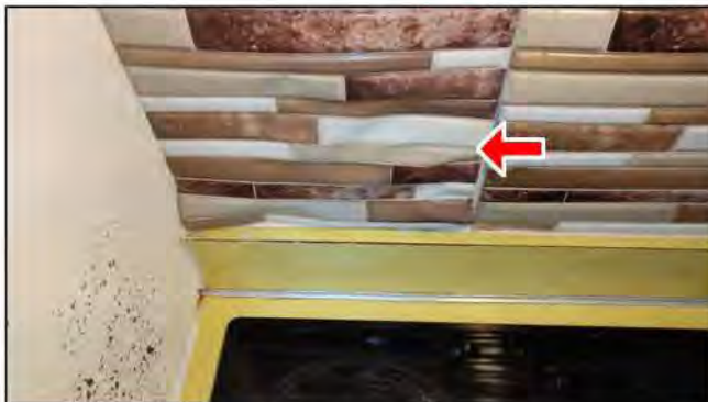
4.1 Item 2(Picture) Stick on tile are loose
