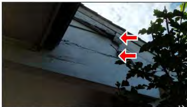
2.0 Item 5(Picture) Deteriorated siding and trim
