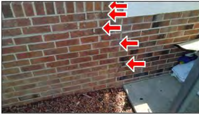
1.0 Item 1(Picture) Long cracking in the brickwork
