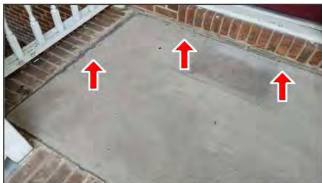
2.5 Item 4(Picture) Front porch has settled and is slopped towards the home
