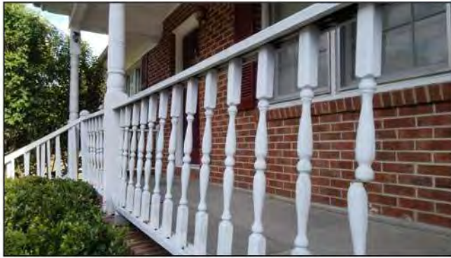
2.5 Item 1(Picture) Loose deteriorated rails and pickets
