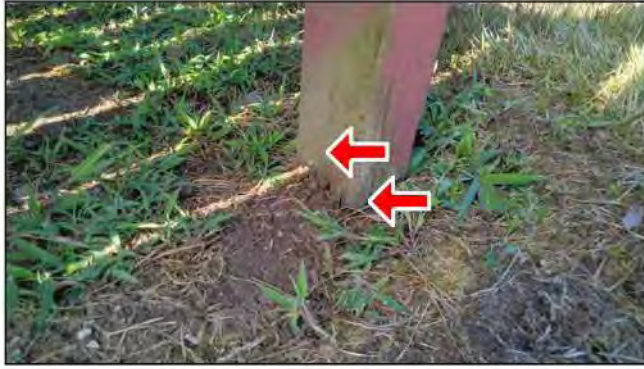
2.8 Item 11(Picture) Deteriorated deck posts
