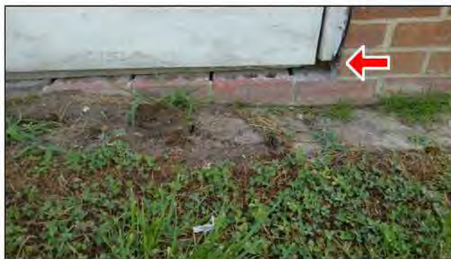
1.3 Item 3(Picture) Gaps at the crawlspace door
