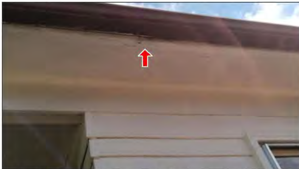
2.1 Item 1(Picture) Deterioration noted at the front and rear fascia boards
