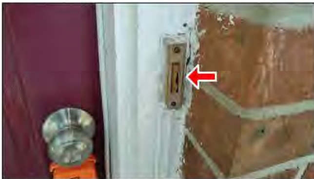
8.11 Item 1(Picture) Broken door bell cover
