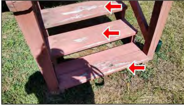
2.8 Item 5(Picture) Deck and steps need to be cleaned and sealed
