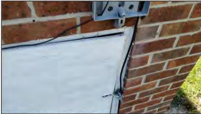
1.3 Item 2(Picture) Gaps at the crawlspace door
