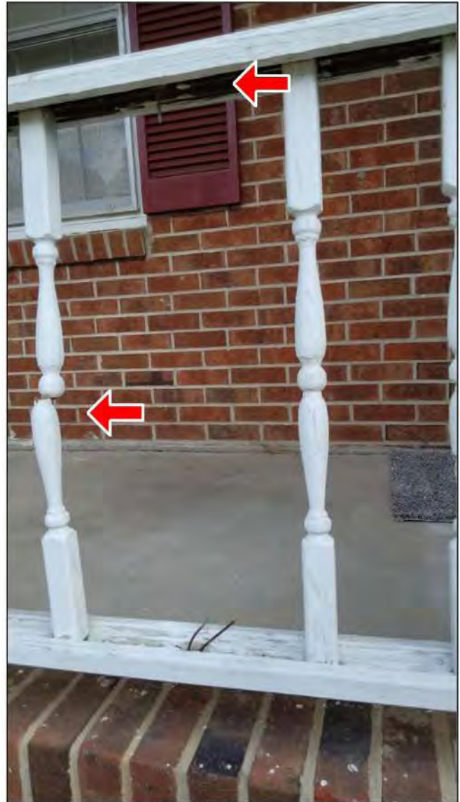
2.5 Item 2(Picture) broken and missing pickets
