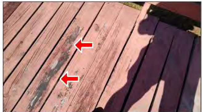
2.8 Item 10(Picture) Deteriorated deck boards
