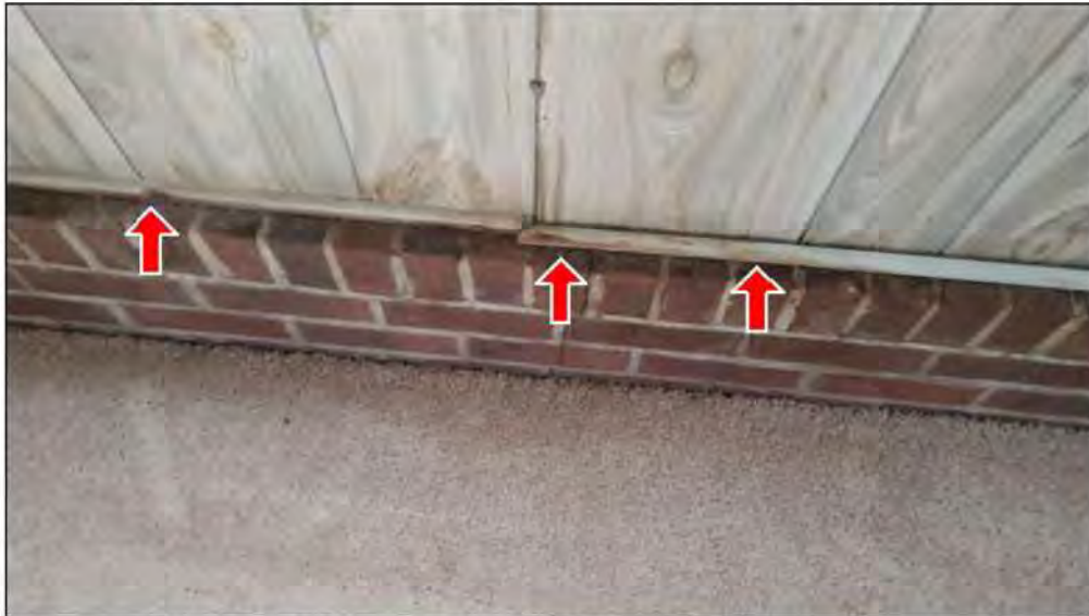
4.7 Item 2(Picture) Moisture stains noted
