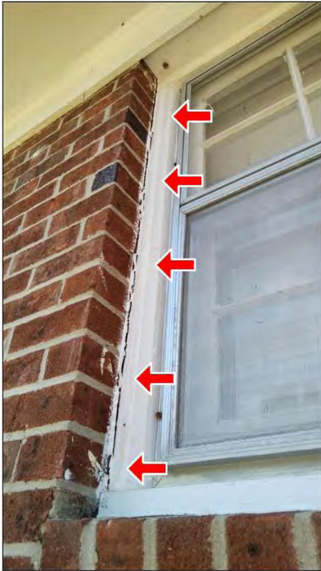
2.2 Item 8(Picture) Caulk has failed
