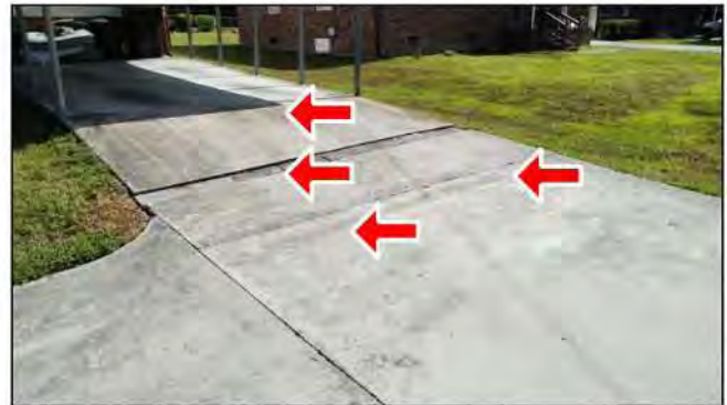
2.7 Item 2(Picture) Common cracks noted
