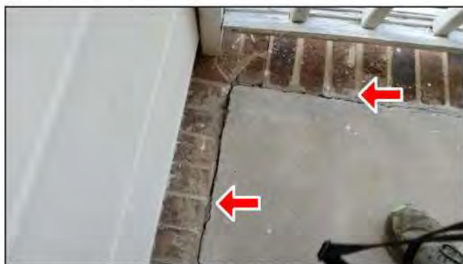
2.5 Item 6(Picture) Outer brickwork is higher than the concrete and will hold water
