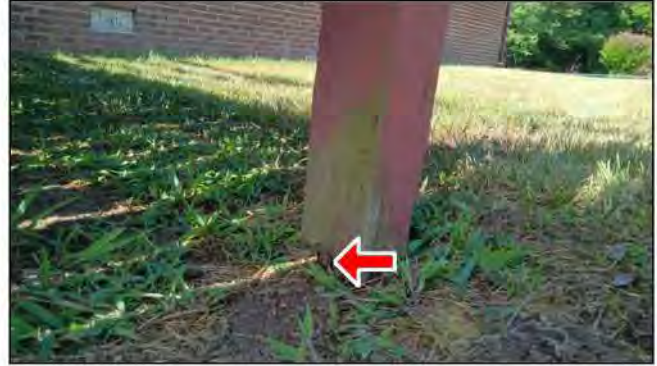
2.8 Item 12(Picture) Deterioration noted at grade
