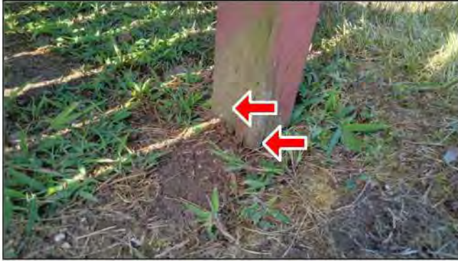
2.8 Item 11(Picture) Deteriorated deck posts
