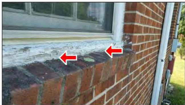
2.2 Item 5(Picture) Failing paint at the windows
