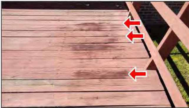
2.8 Item 9(Picture) Deteriorated decking boards
