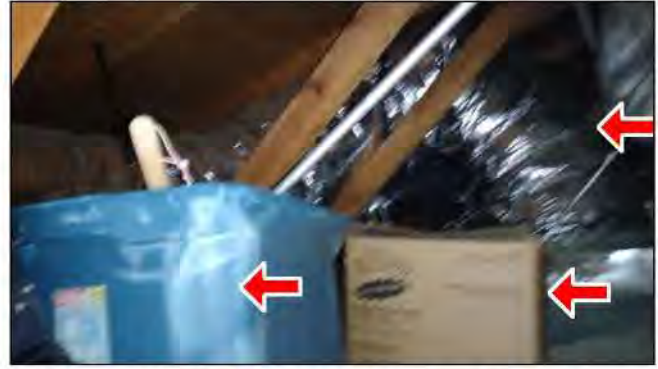
1.8 Item 2(Picture) Stored items in the attic
