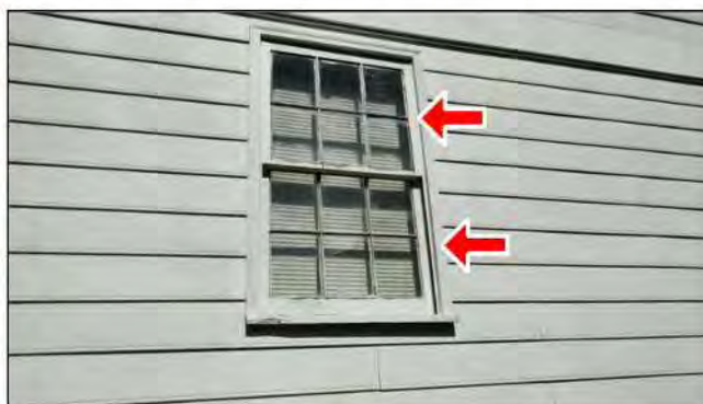
2.3 Item 4(Picture) Missing storm window
