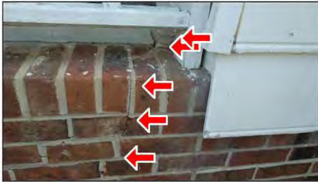
1.0 Item 3(Picture) Structural crack has settlement in the front porch noted
