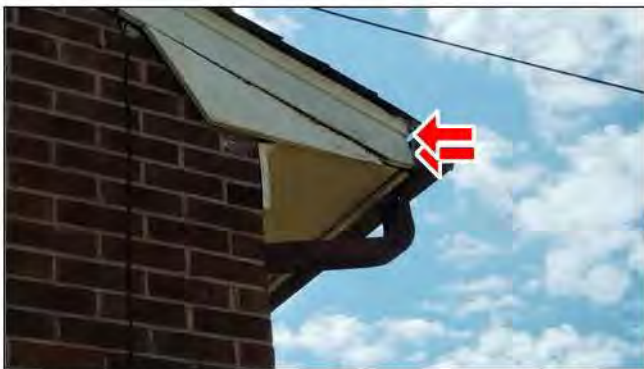
2.1 Item 2(Picture) Deterioration noted in the rake boards
