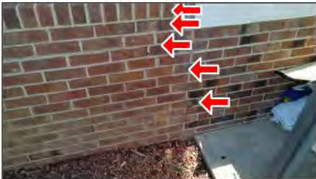
1.0 Item 1(Picture) Long cracking in the brickwork
