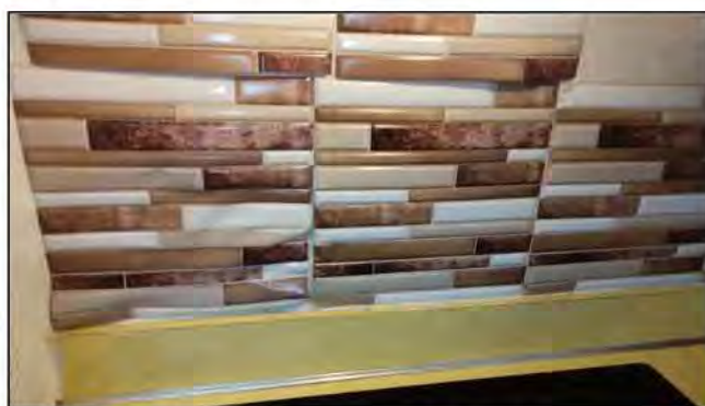
4.1 Item 3(Picture) Stick on tile are loose
