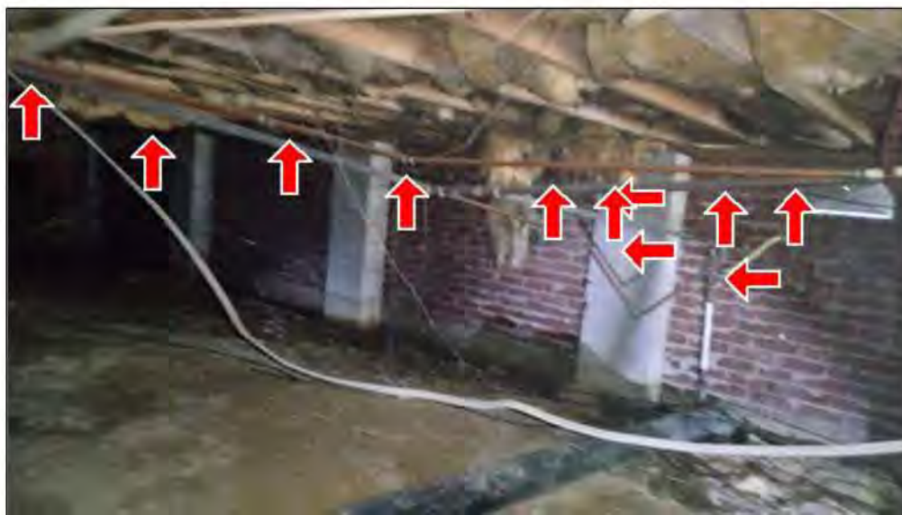
5.1 Item 1(Picture) Water supply lines not strapped or supported
