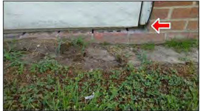
1.3 Item 3(Picture) Gaps at the crawlspace door
