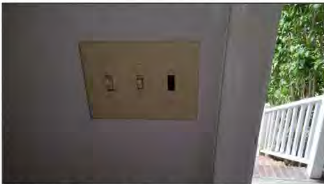
8.7 Item 1(Picture) Switch missing leaving exposed wiring
