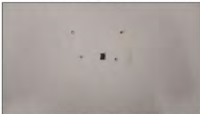
4.1 Item 1(Picture) Holes and damage in the wall
