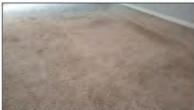
4.2 Item 1(Picture) Loose carpet noted
