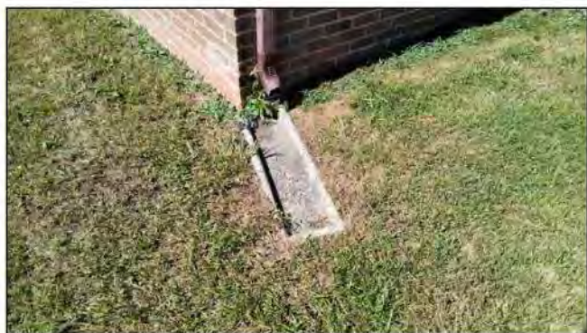
3.1 Item 1(Picture) water draining back against the home
