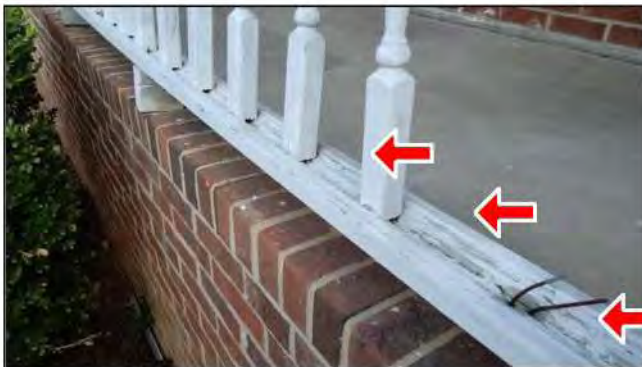
2.5 Item 3(Picture) Deteriorated railing and pickets
