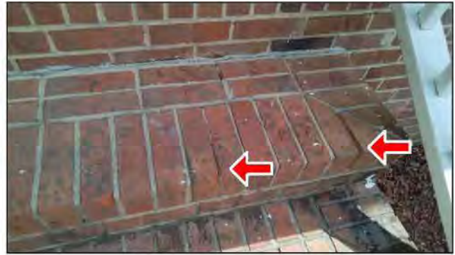
2.6 Item 2(Picture) Missing mortar noted
