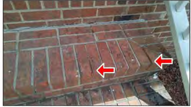
2.6 Item 2(Picture) Missing mortar noted
