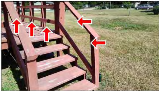
2.8 Item 13(Picture) Improperly spaced pickets
