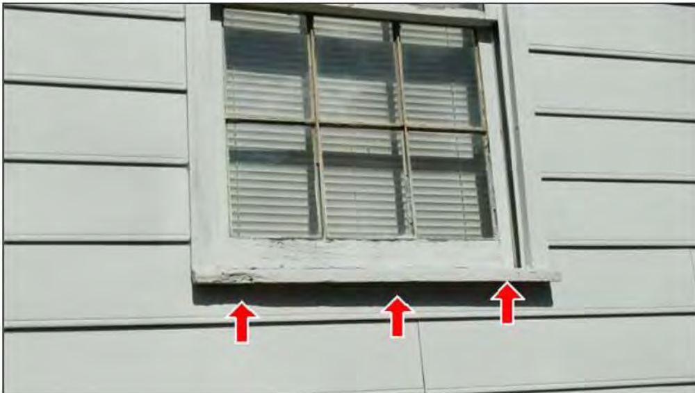
2.2 Item 7(Picture) Failing paint on the windows
