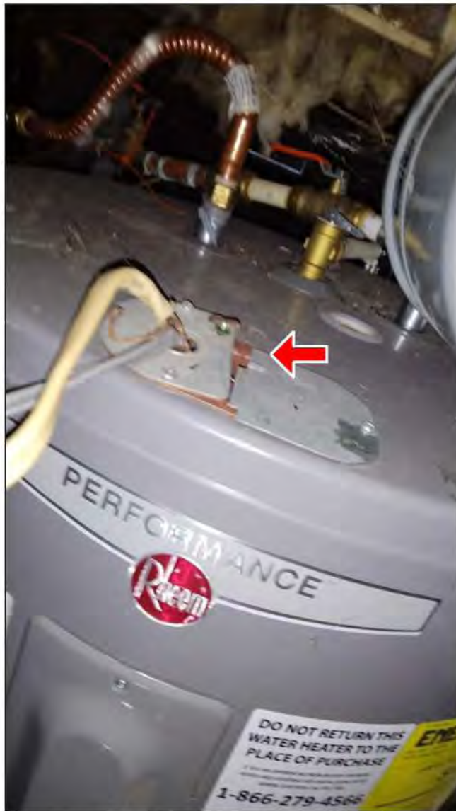
6.3 Item 1(Picture) Wiring not properly connected
