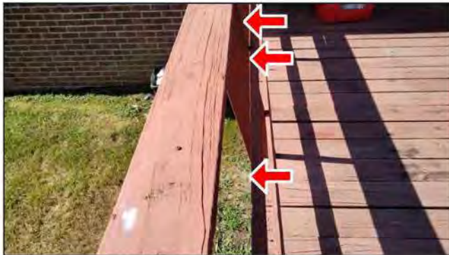
2.8 Item 7(Picture) Splintering hand rails
