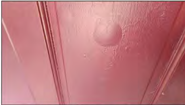
2.2 Item 3(Picture) Bubbling paint on the front door
