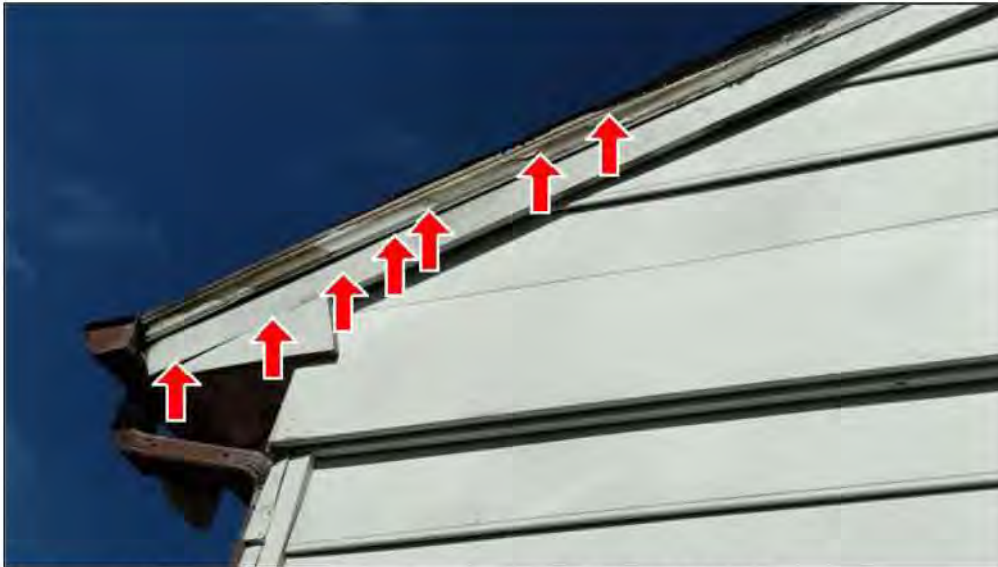
3.0 Item 2(Picture) Shingles are not covering the drip edge
