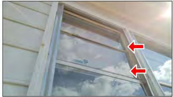
2.4 Item 2(Picture) broken glass
