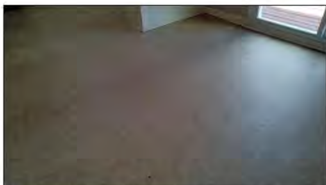
4.2 Item 2(Picture) Large dip noted in the kitchen floor
