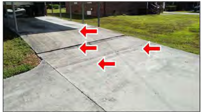
2.7 Item 2(Picture) Common cracks noted
