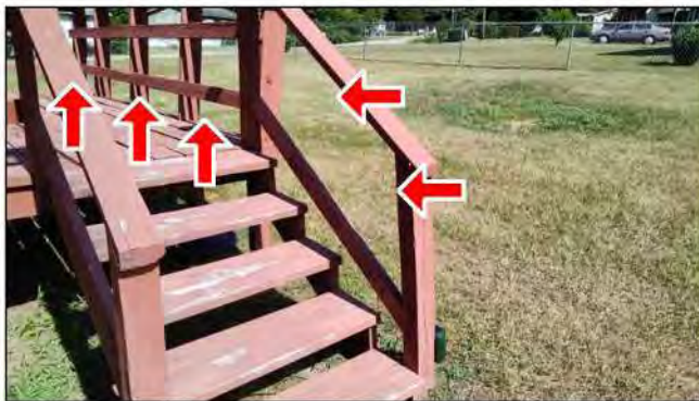
2.8 Item 13(Picture) Improperly spaced pickets
