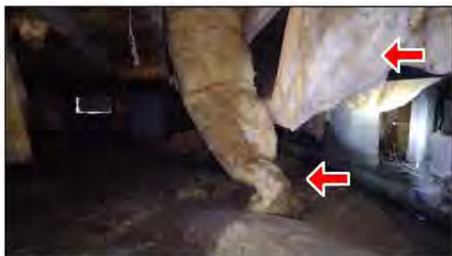
11.1 Item 1(Picture) The flooring insulation has fallen in areas of the crawlspace
