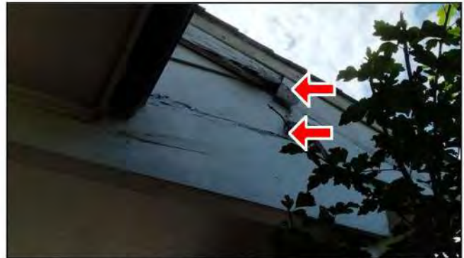
2.0 Item 5(Picture) Deteriorated siding and trim
