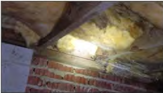
1.2 Item 2(Picture) Heavy fungal growth on the floor framing
