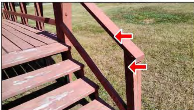
2.8 Item 4(Picture) Loose hand rail
