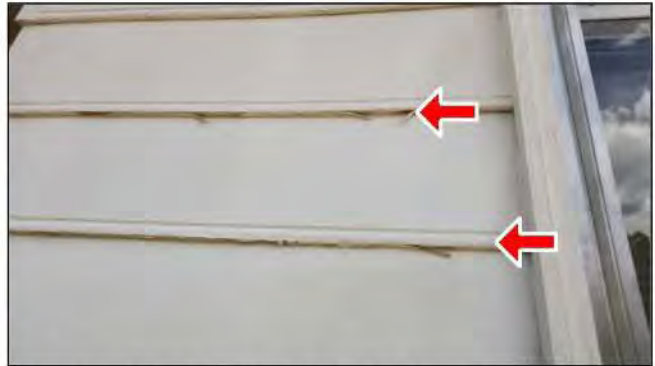
2.2 Item 9(Picture) Failing paint noted on the siding
