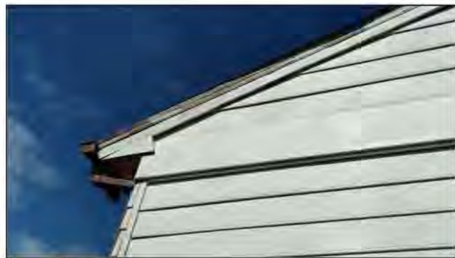
3.0 Item 1(Picture) Shingles are not covering the drip edge or trim
