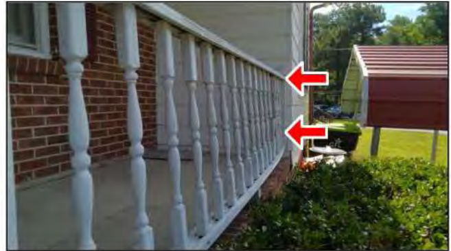
2.2 Item 2(Picture) failing paint on front porch rail
