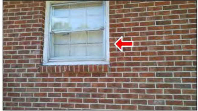
2.3 Item 6(Picture) missing screen
