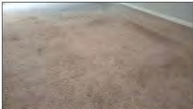
4.2 Item 1(Picture) Loose carpet noted
