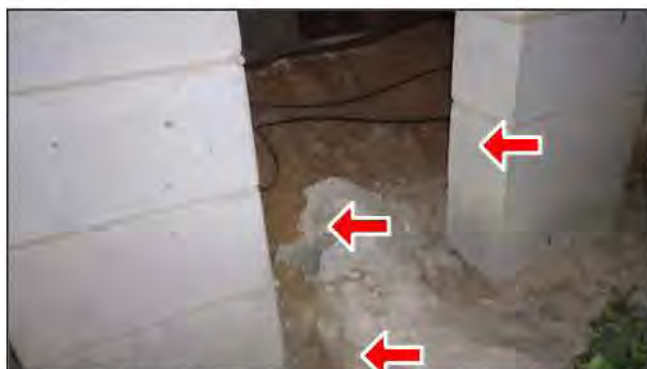
1.1 Item 1(Picture) The foundation piers footers have not been back filled
