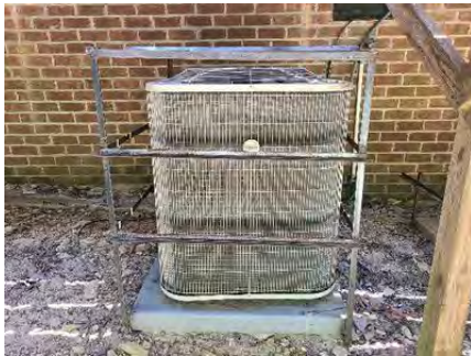
Exterior AC unit 2019 manufacturer date.
